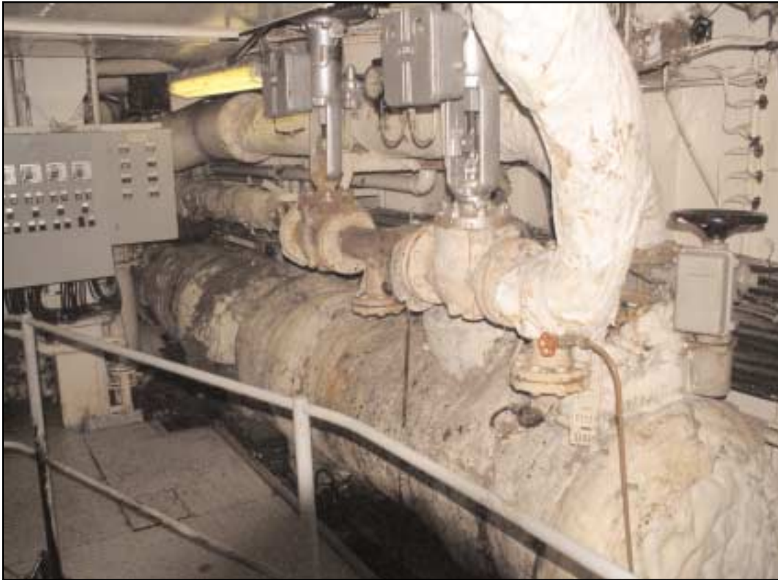
Port and starboard dump condensers
