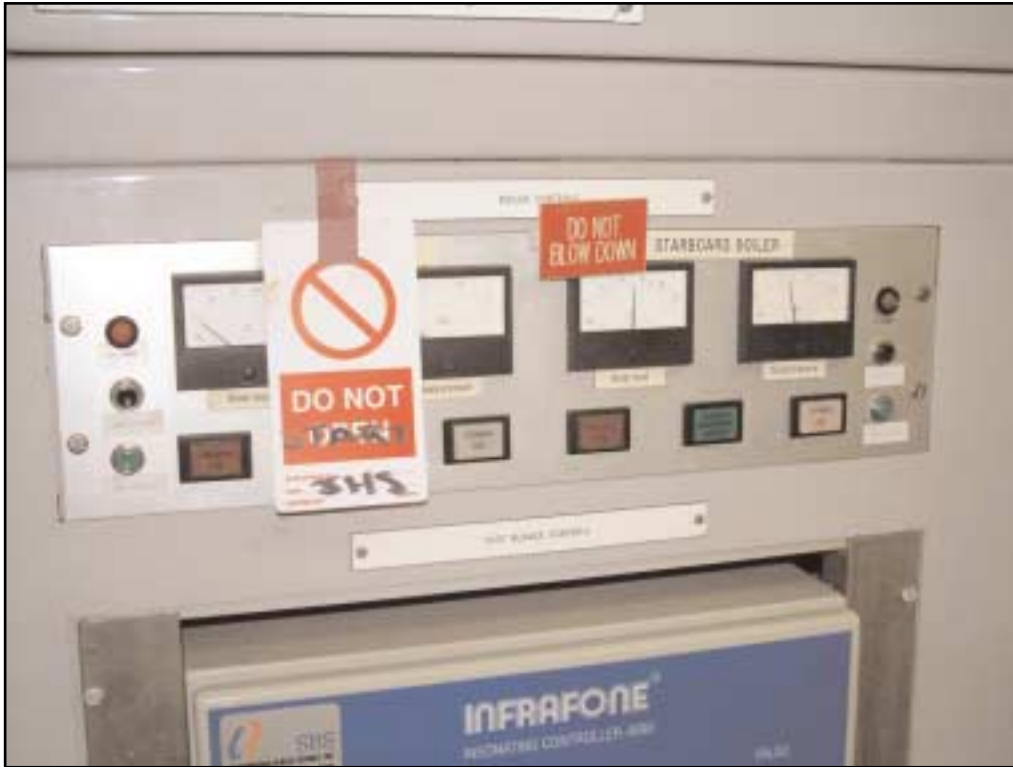
Control room boiler control panel
