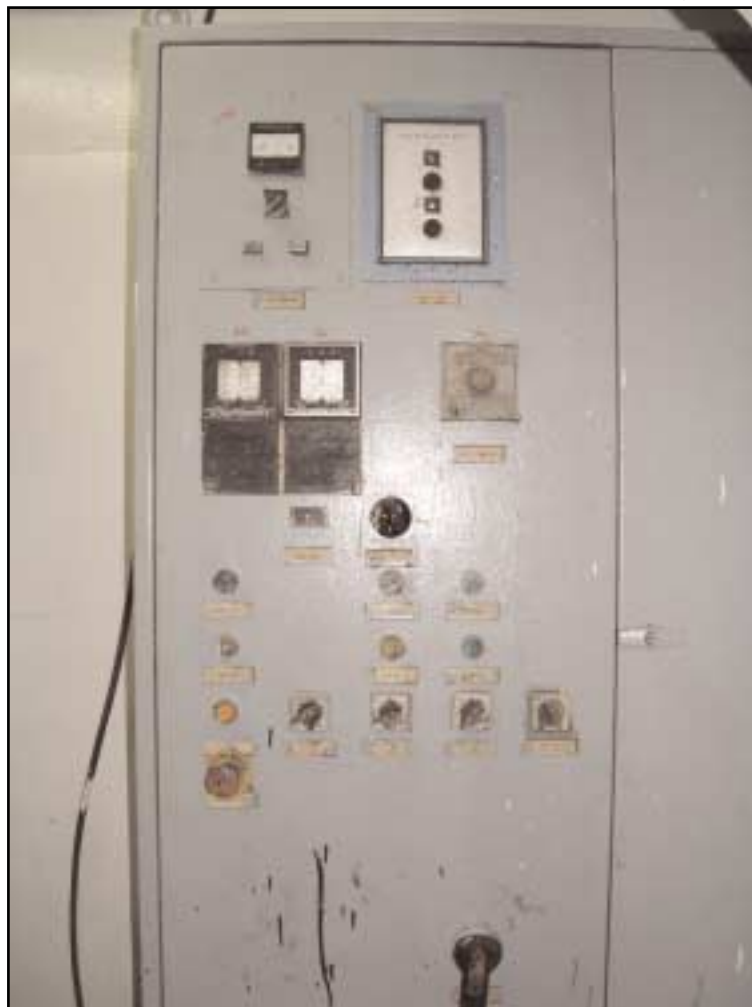
Local boiler control panel
