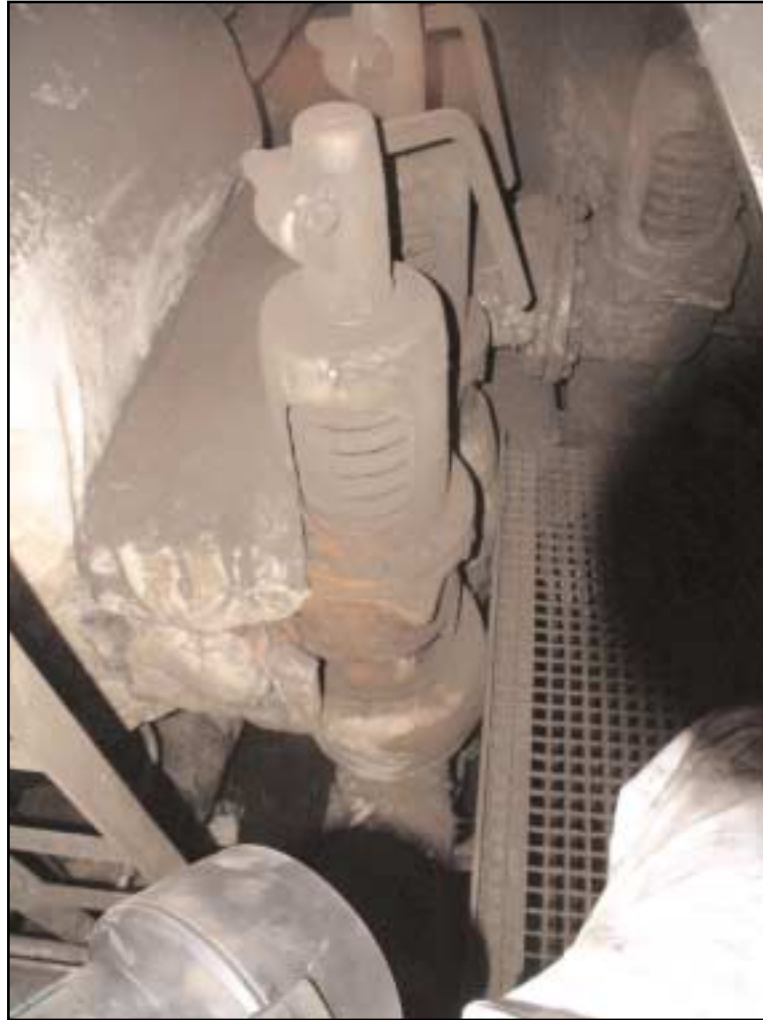
Port system safety valves
