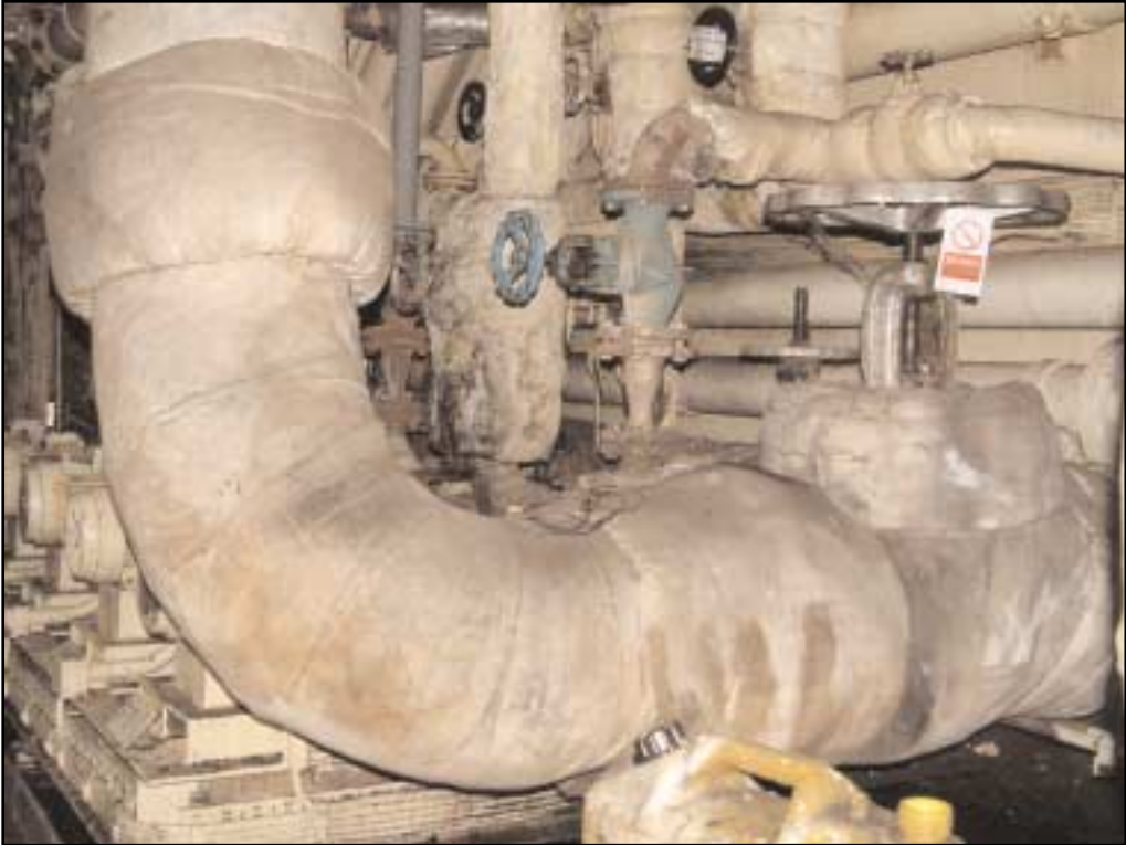
EGB circulating pumps main suction from the port boiler
