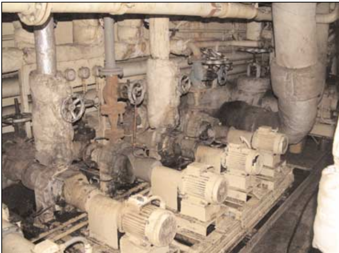
EGB circulating pumps
