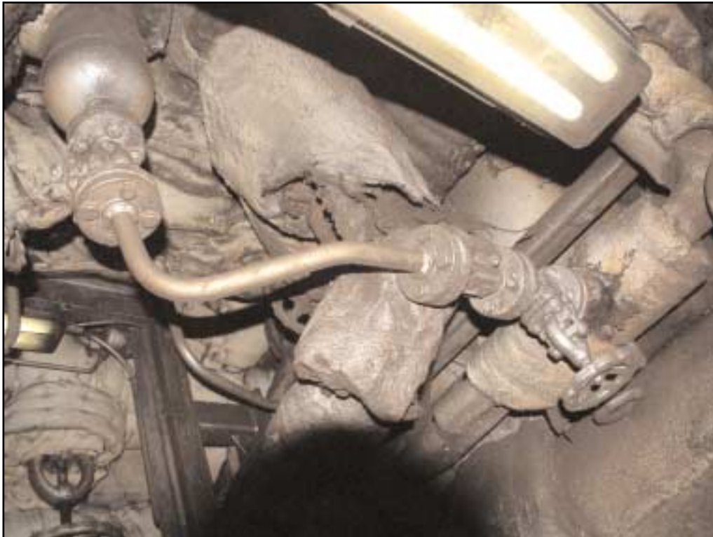
Drain from below port system safety valves
