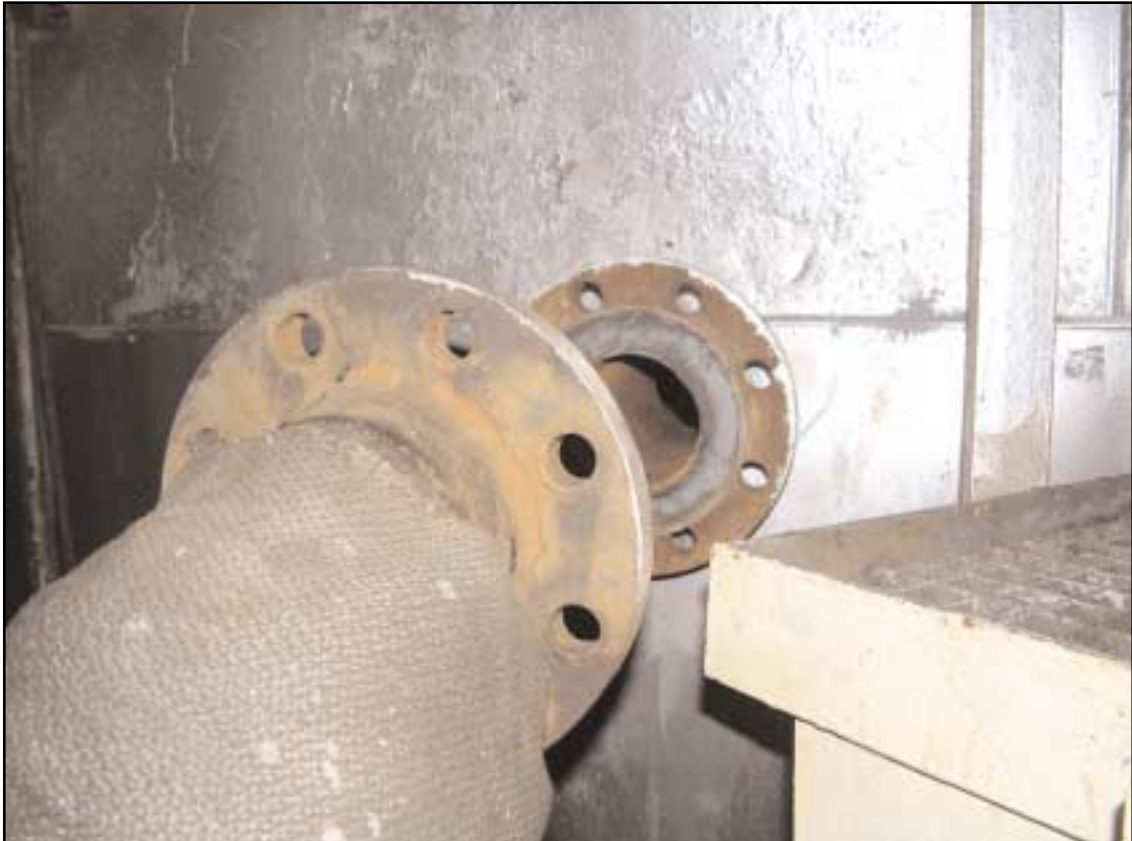
Mounting position for port boiler EGB suction valve
