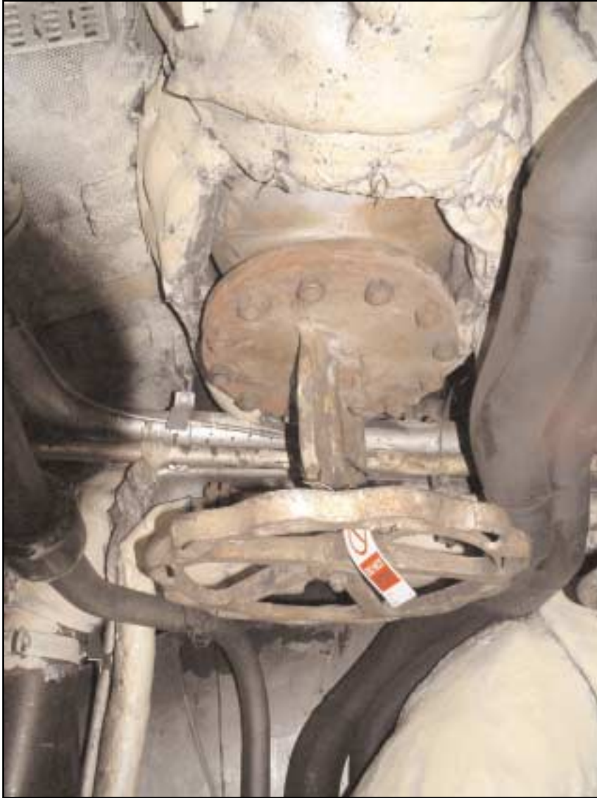
Hotel services steam supply cross-connecting valve
