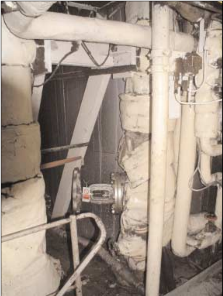
Port boiler supply to the engine room steam ring main
