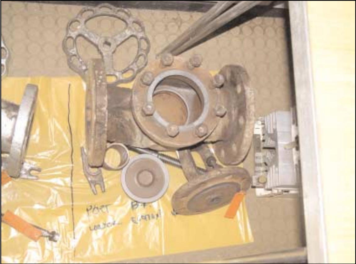
Port boiler EGB suction valve
