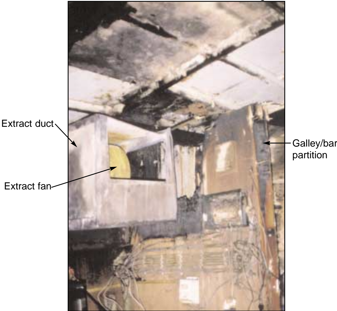
Charring of the wood deckhead, which fell away from the steel supports above the galley extract ductwork
