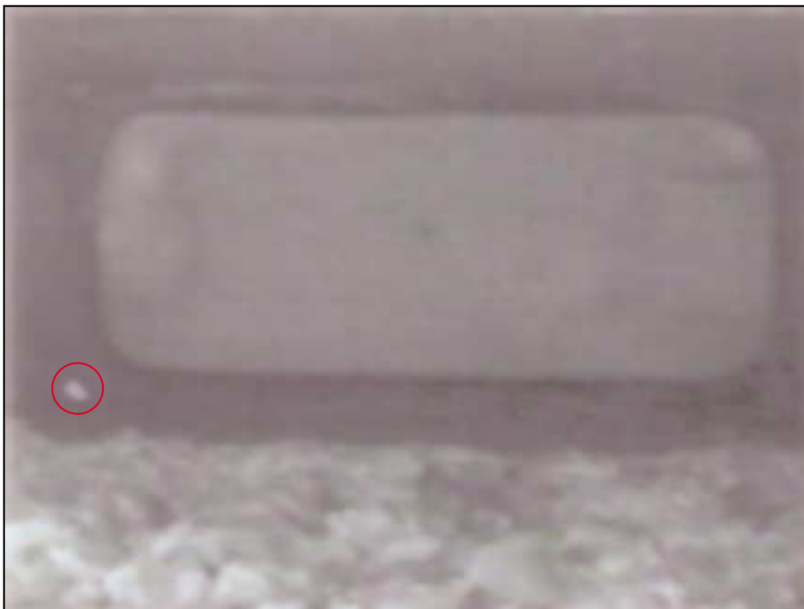
Photograph showing hole at the top of the propeller inspection port
