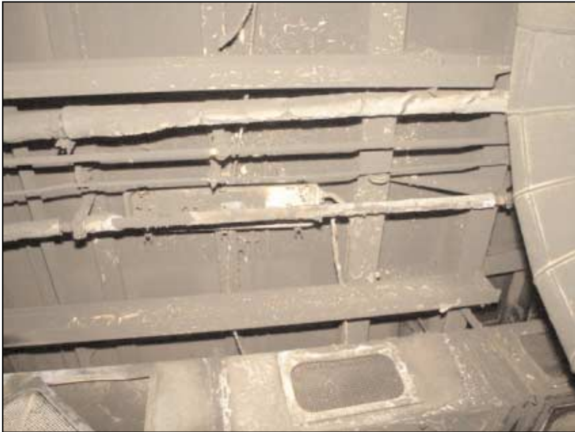
Deckhead and lagging damage
