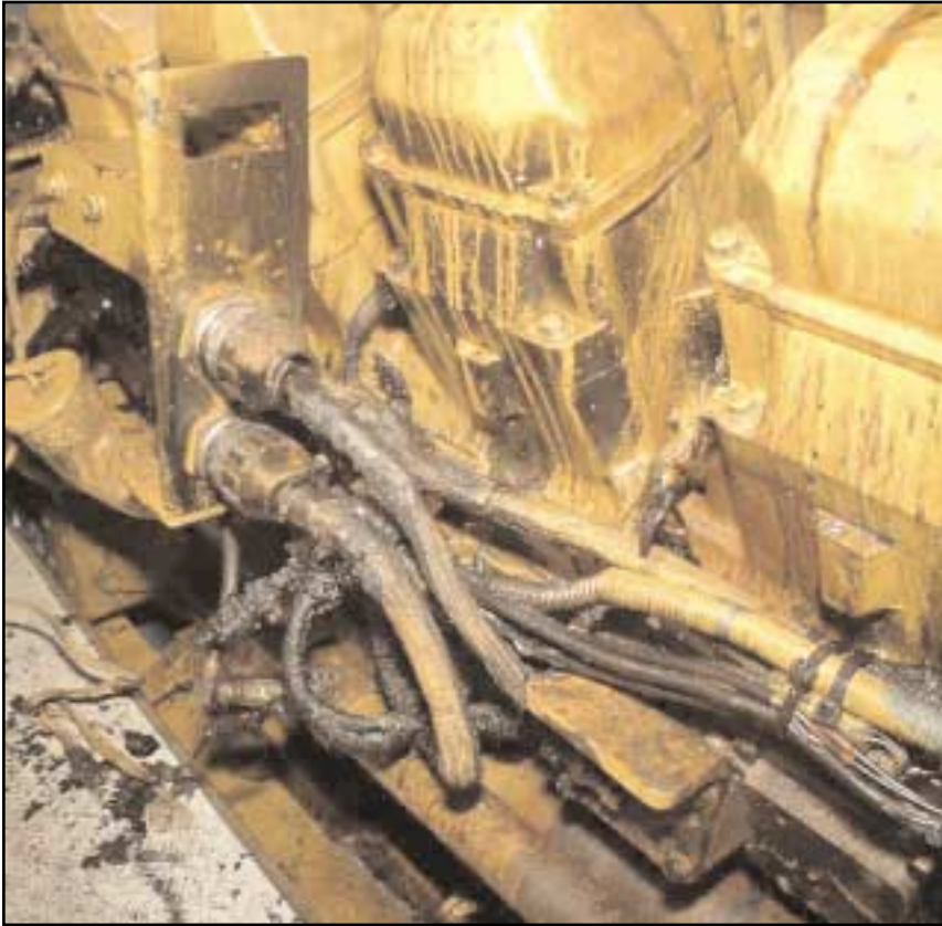
Damage to main engine surveillance and management system electrical loom
