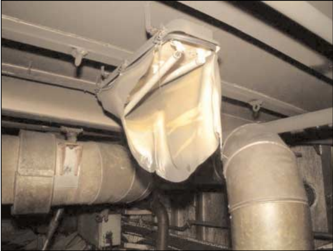
Melted light fittings
