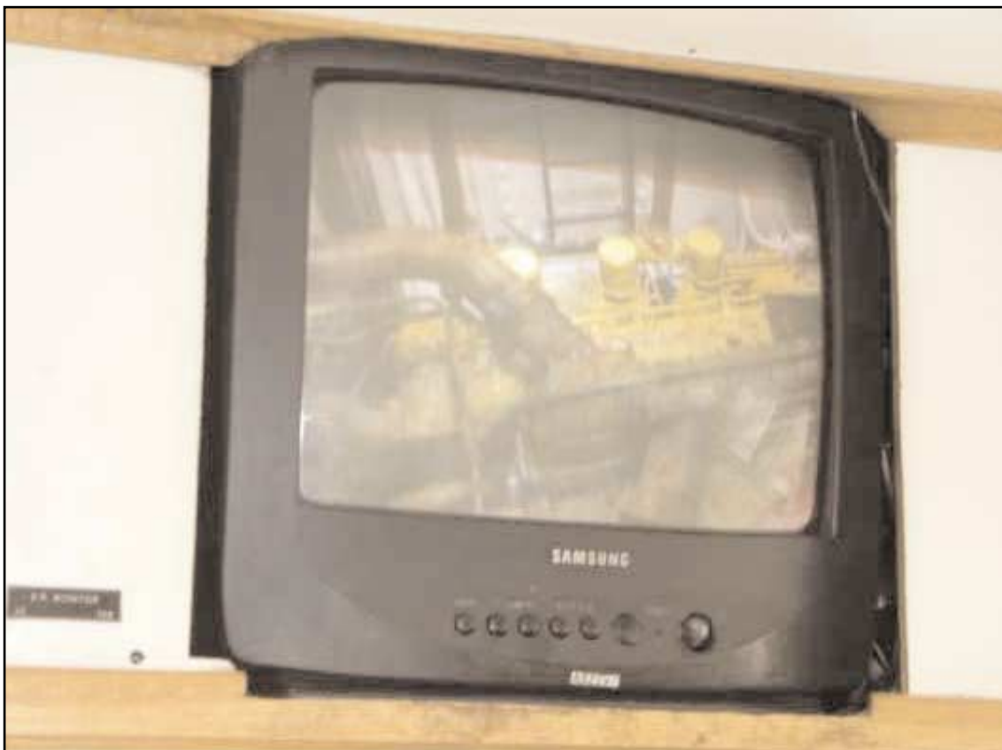
Engine room monitor showing fixed coverage
