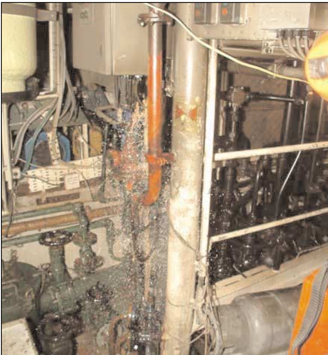
Replicated fuel leakage from main engine duplex fuel filters
