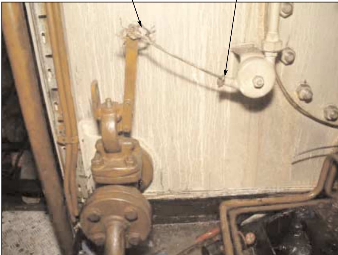
Daily tank quick acting fuel oil shut off valve arrangement
