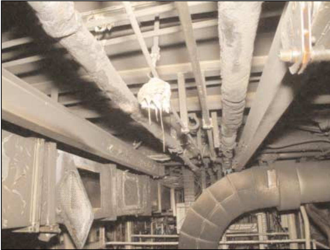
Ventilation trunking and smoke detector damage
