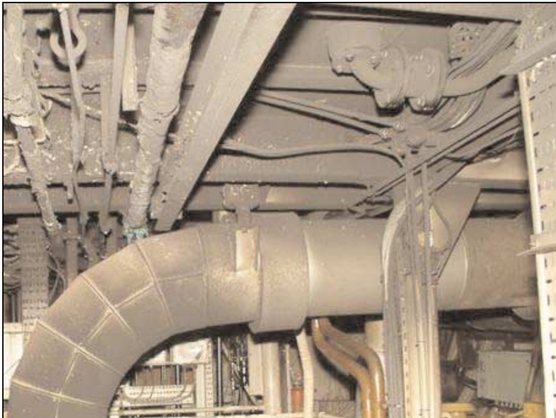
General deckhead damage
