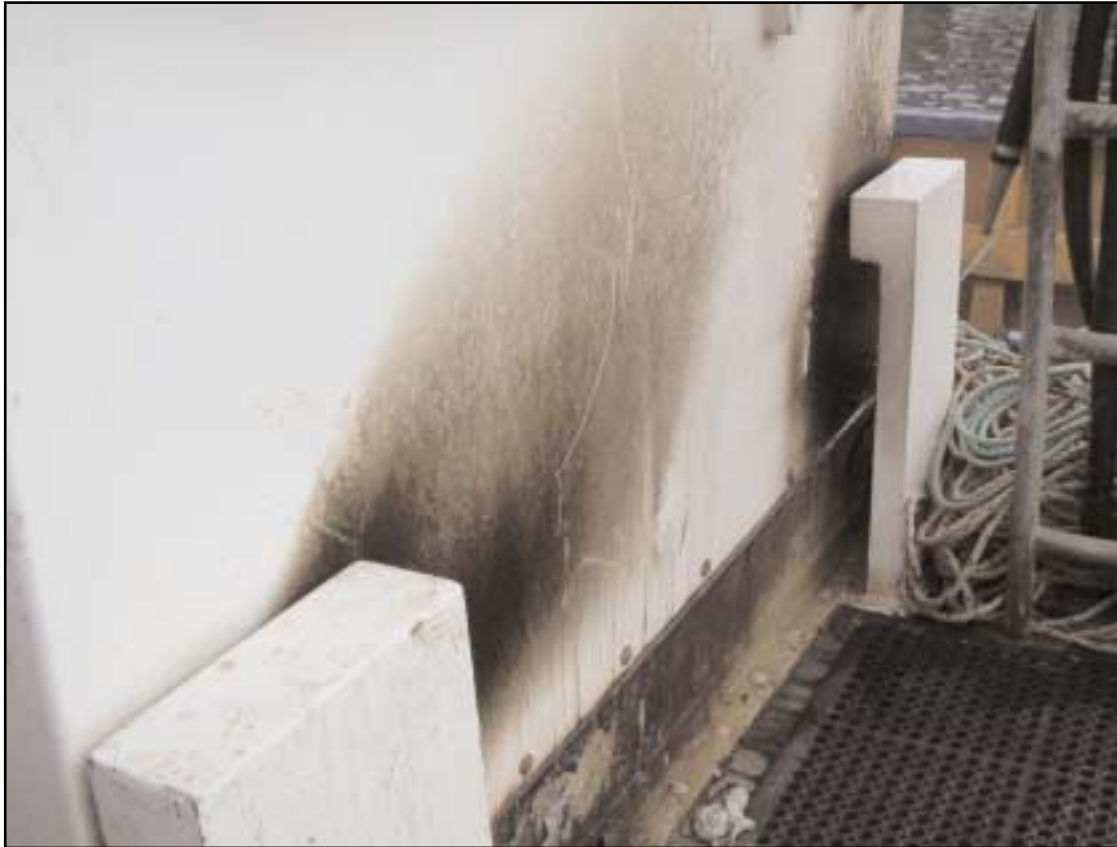
Smoke discharge marks from engine room vents
