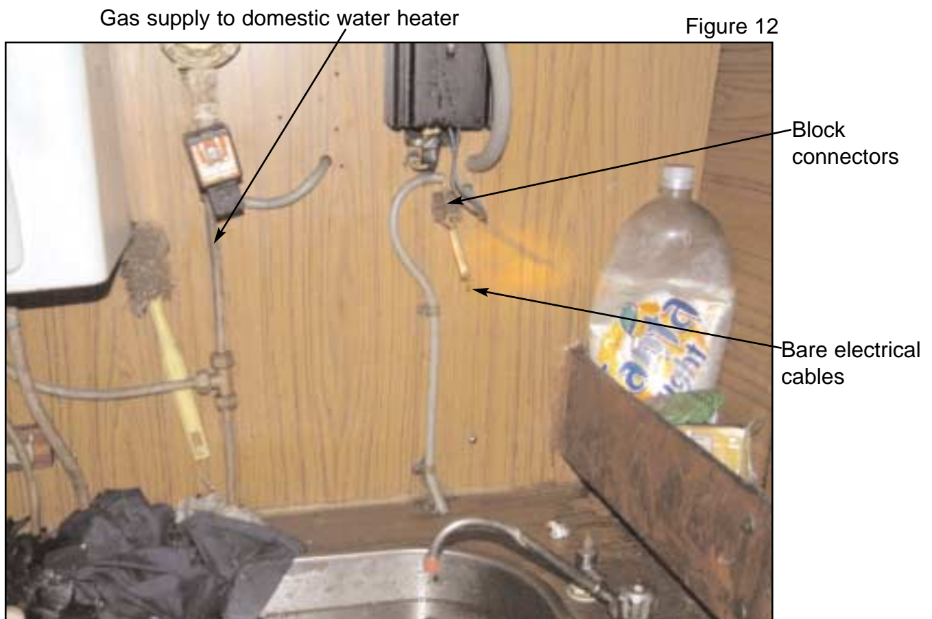
Example of block connector use and exposed wiring
