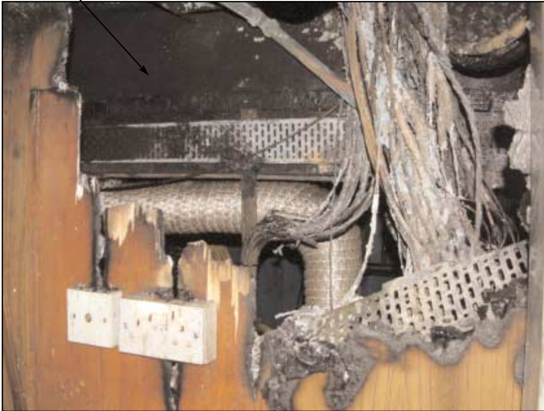
Site of distribution box
