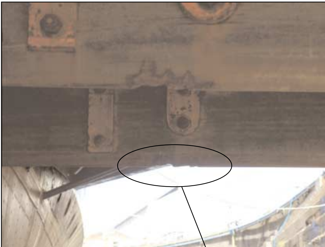
Damage to port side paddle floats
