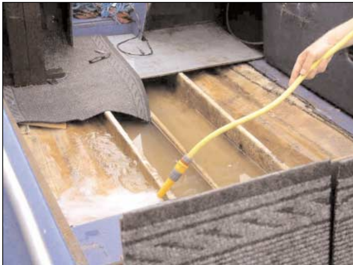
Void filled with water
