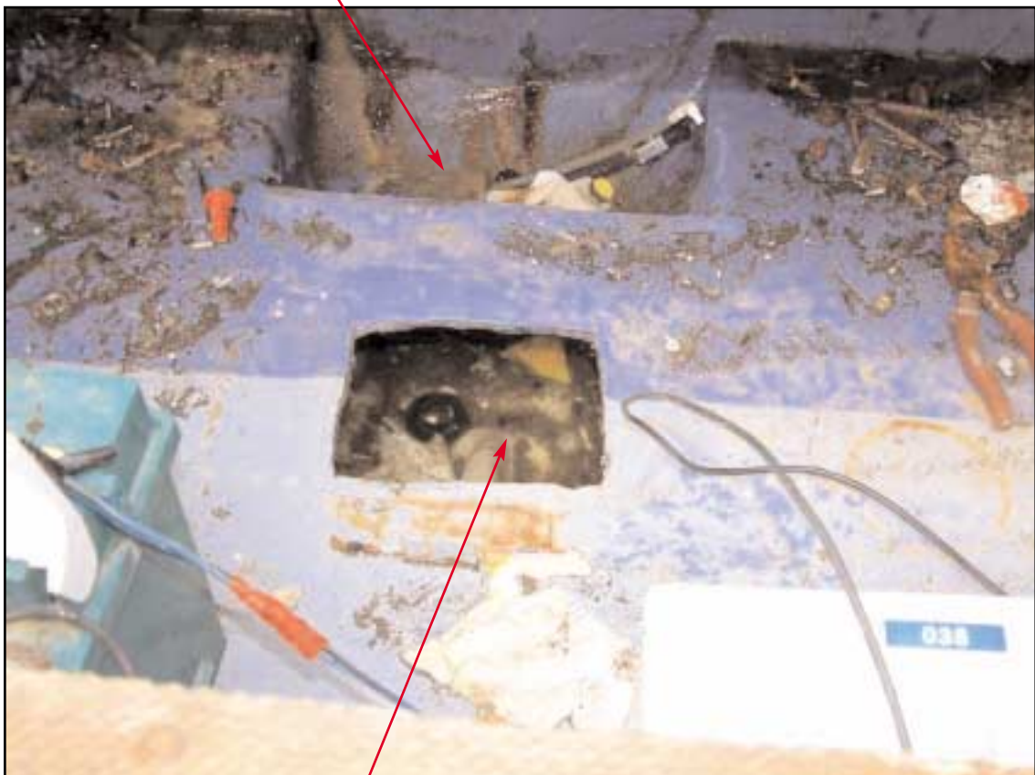
The opening cut in the top of the void at the aft end
