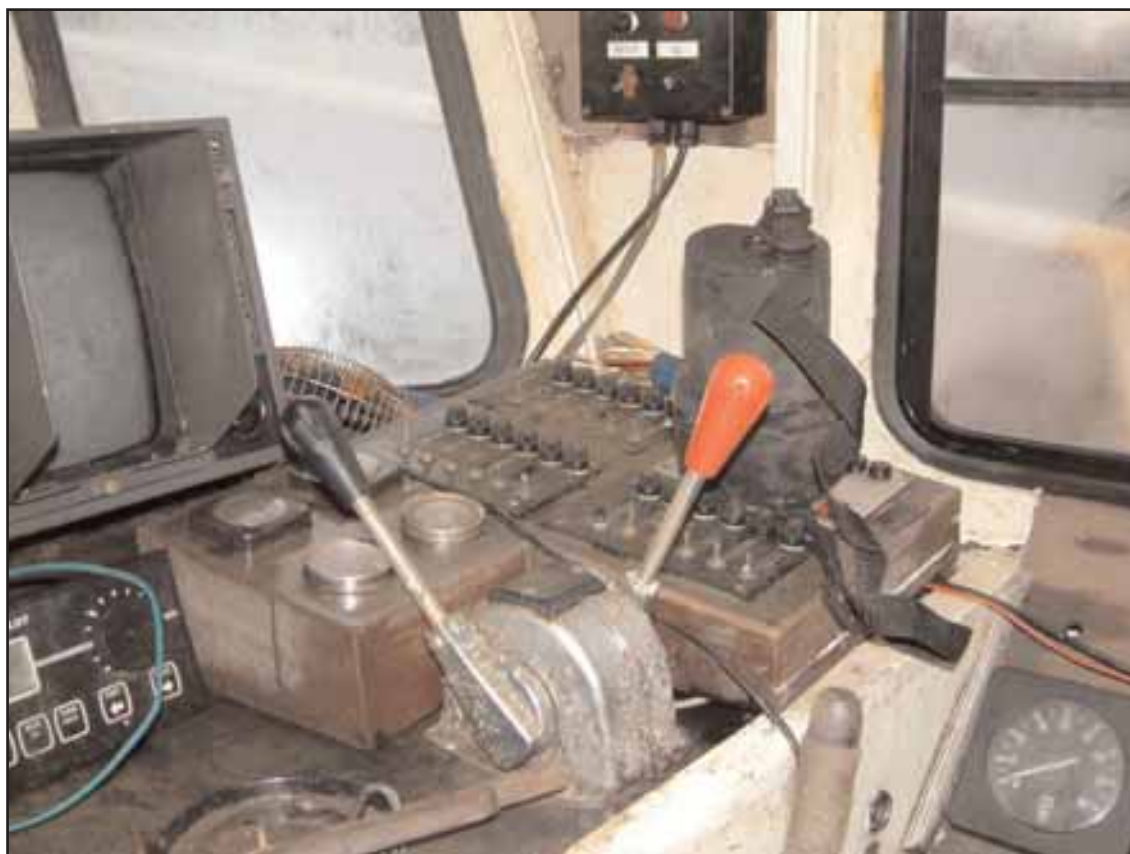
Wheelhouse engine and gearbox control levers
