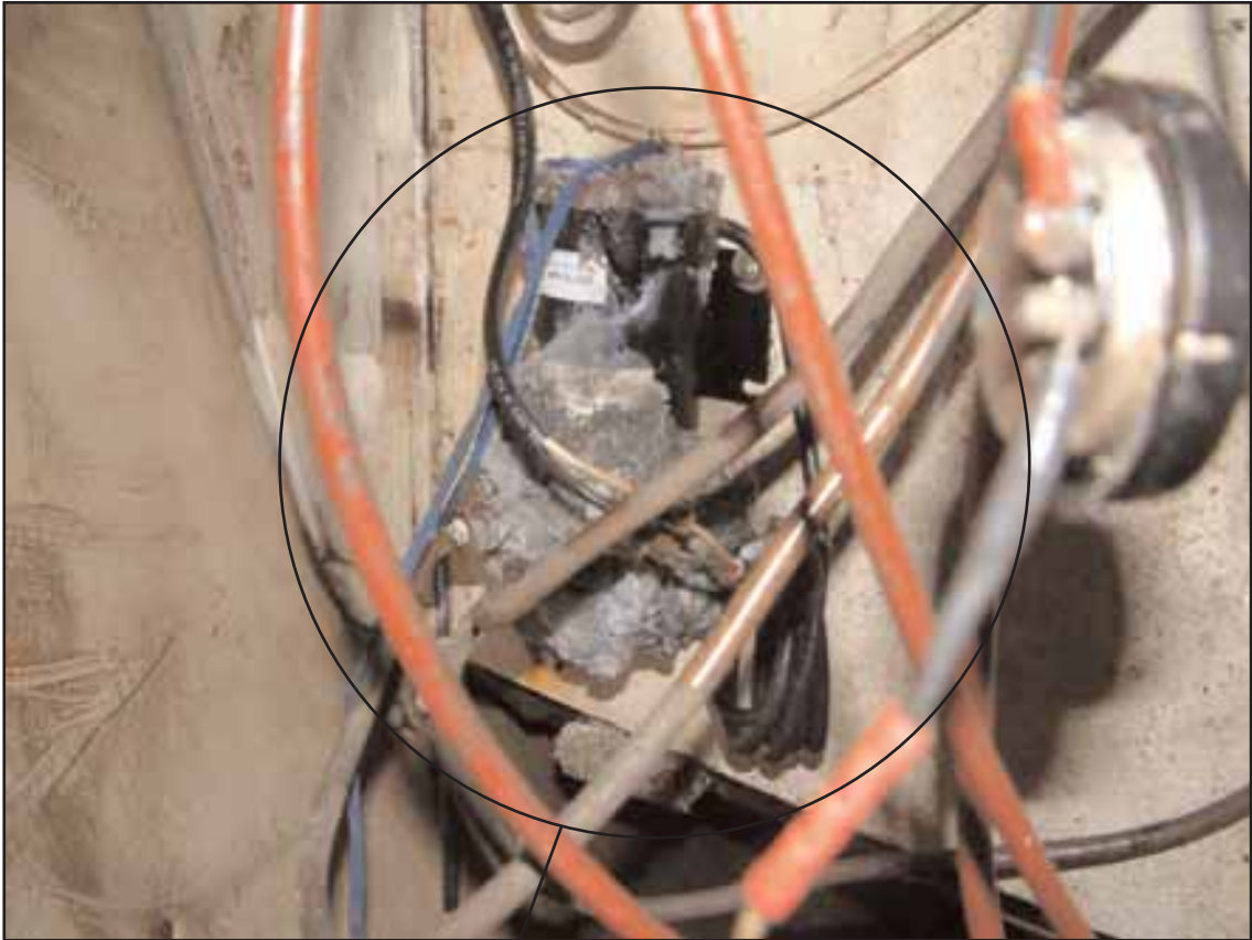
Steering gear hydraulic pump arrangement
