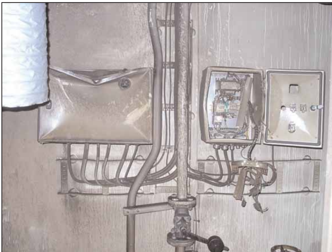
Damage in bow thruster room
