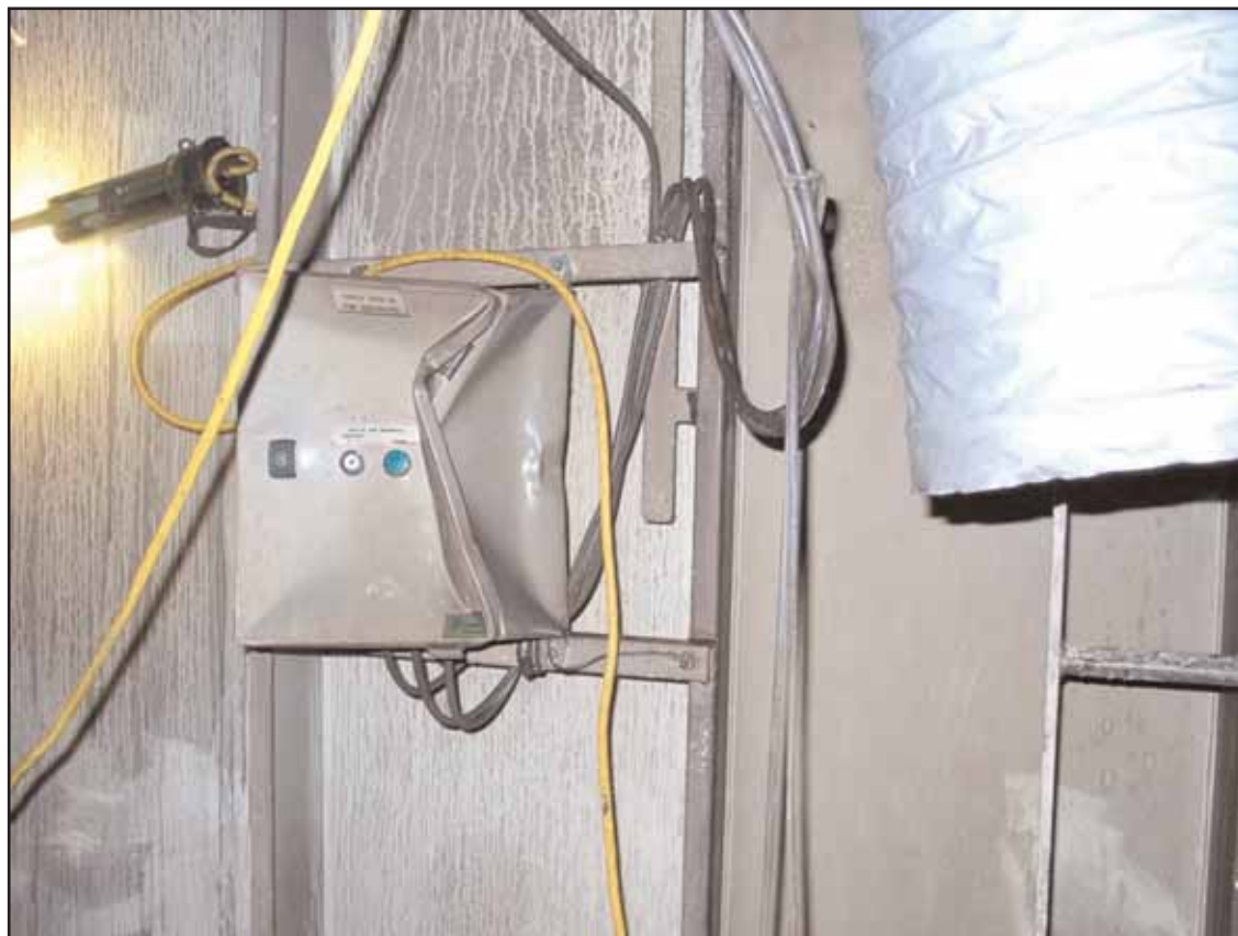
Damage in bow thruster room
