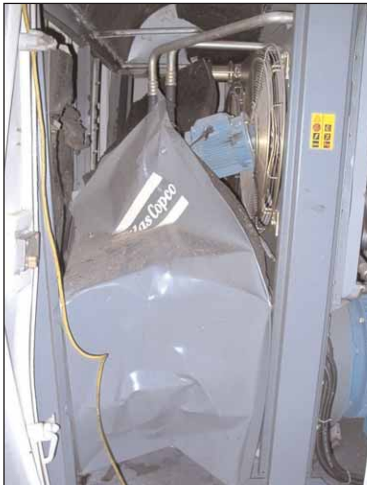
Pressure damage to compressor enclosure
