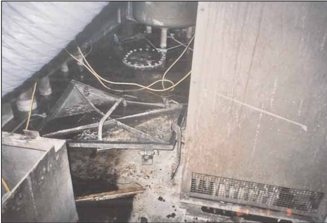
Damage to hatch
