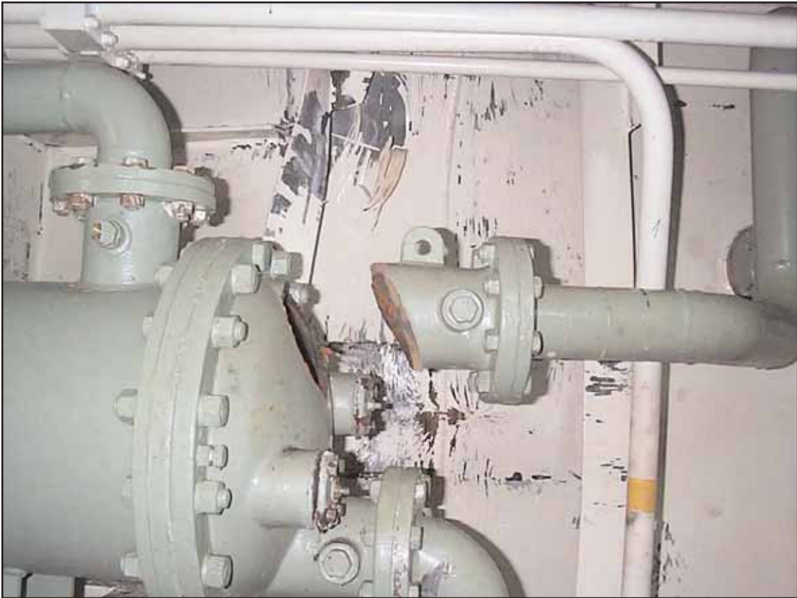
Damage to the starboard main engine jacket water cooling heat exchanger and ships side
