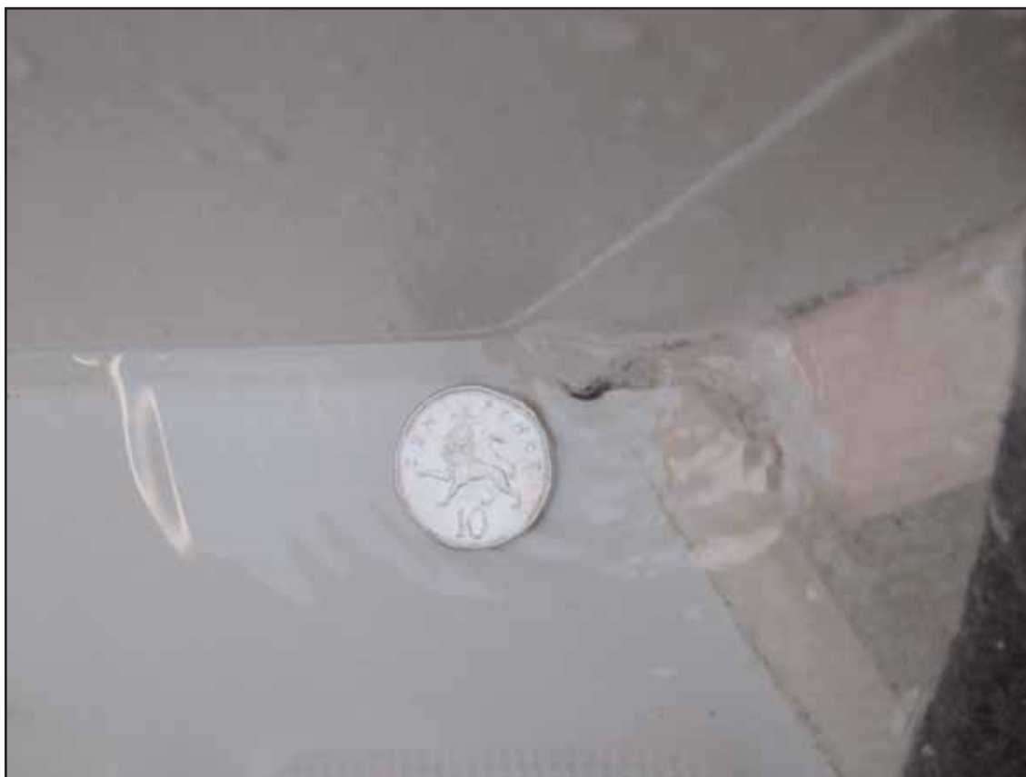
Water passing through deck seam
