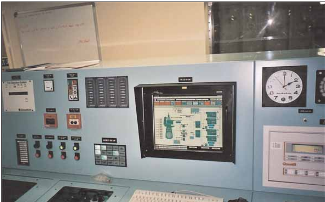
Main Operating Panel (MOP)
