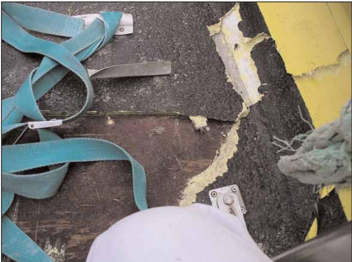
Failure of CSM over deck butt joints
