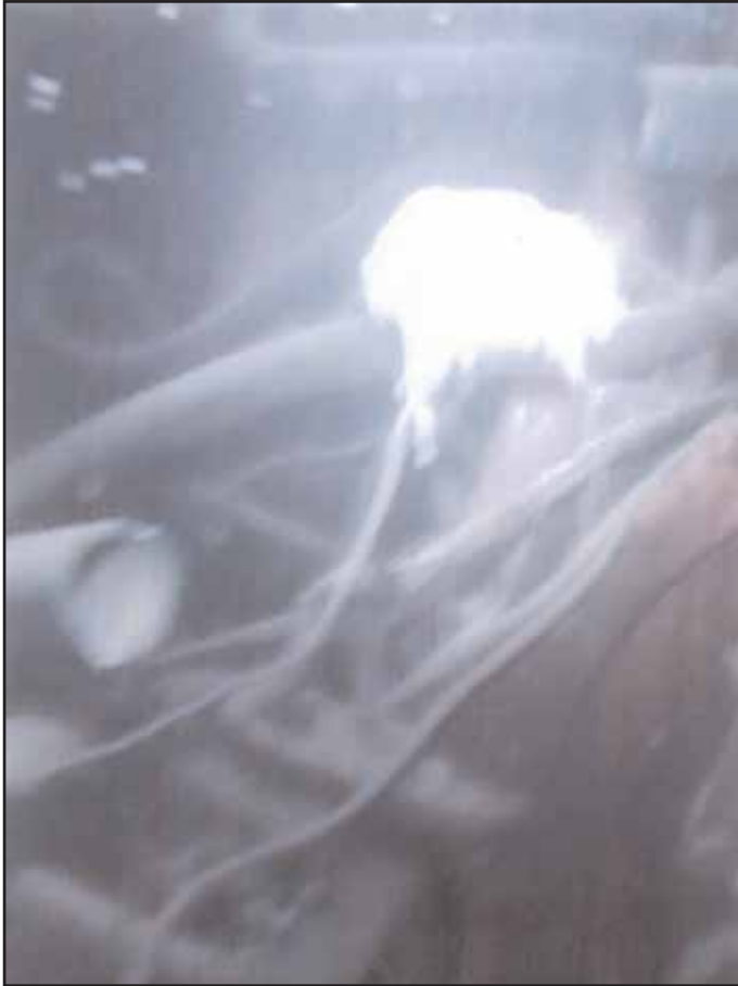
Cut hose in engine sea water system
