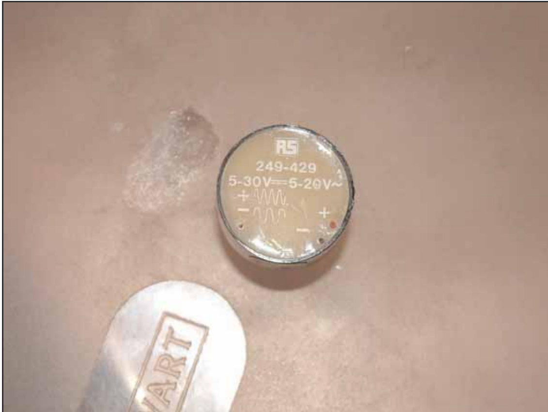
Watch alarm. Buzzer found disconnected.
