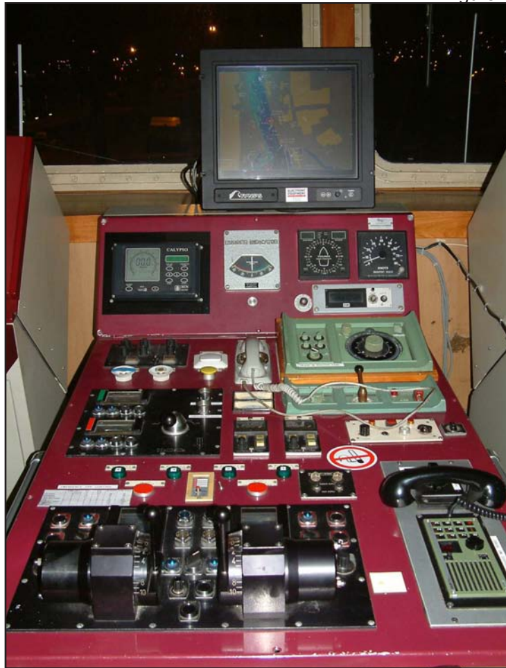
Transas ECS positioned on the centreline
