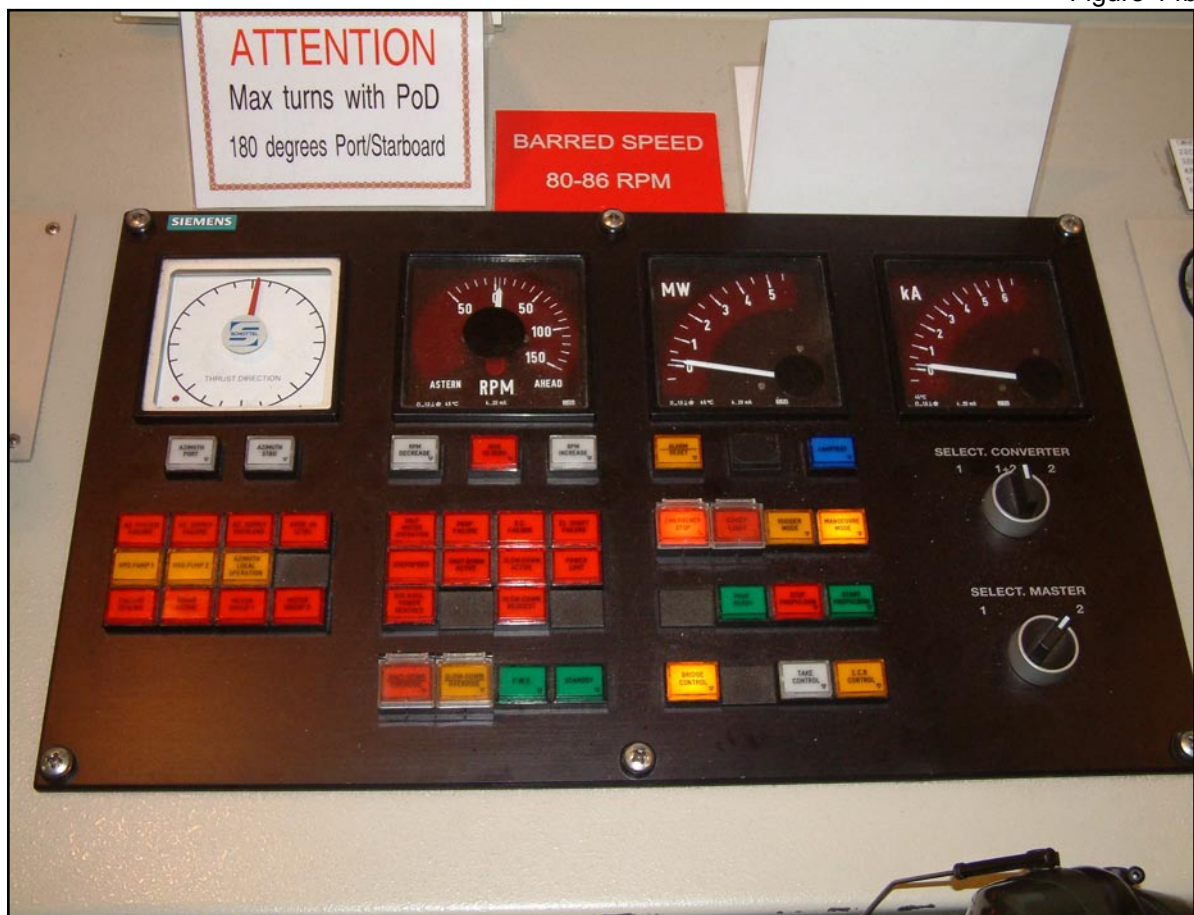
ECR control console, close up showing pod controls.
