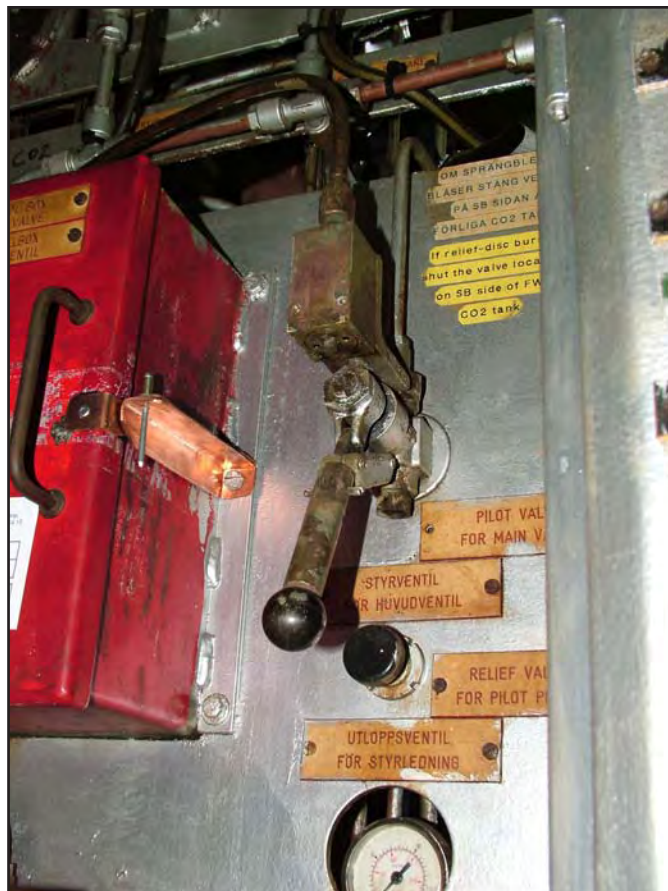
Main pilot release control valve on the CO 2 room control panel
