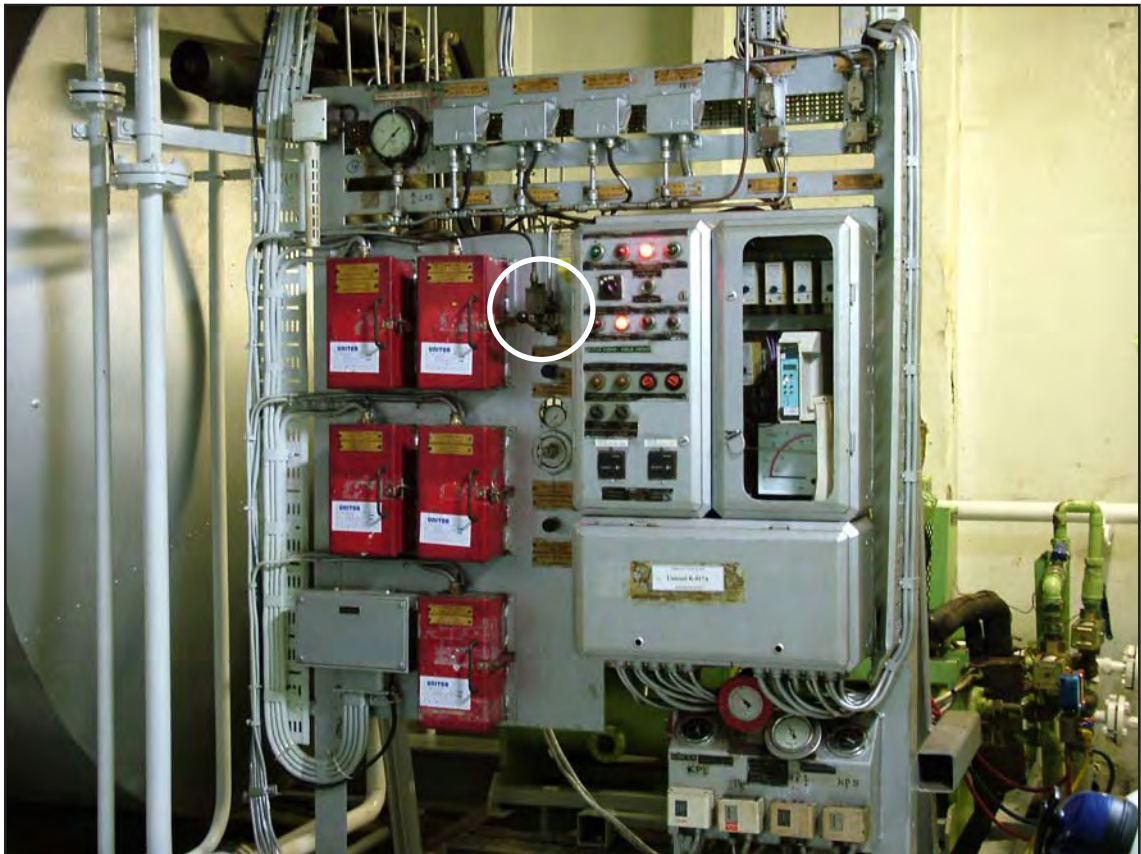
Main release valve in the CO 2 room on Deck 5
