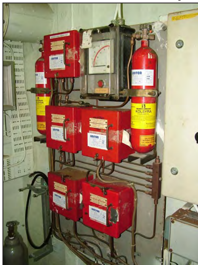
Master Control Unit (MCU) panel on Deck 14
