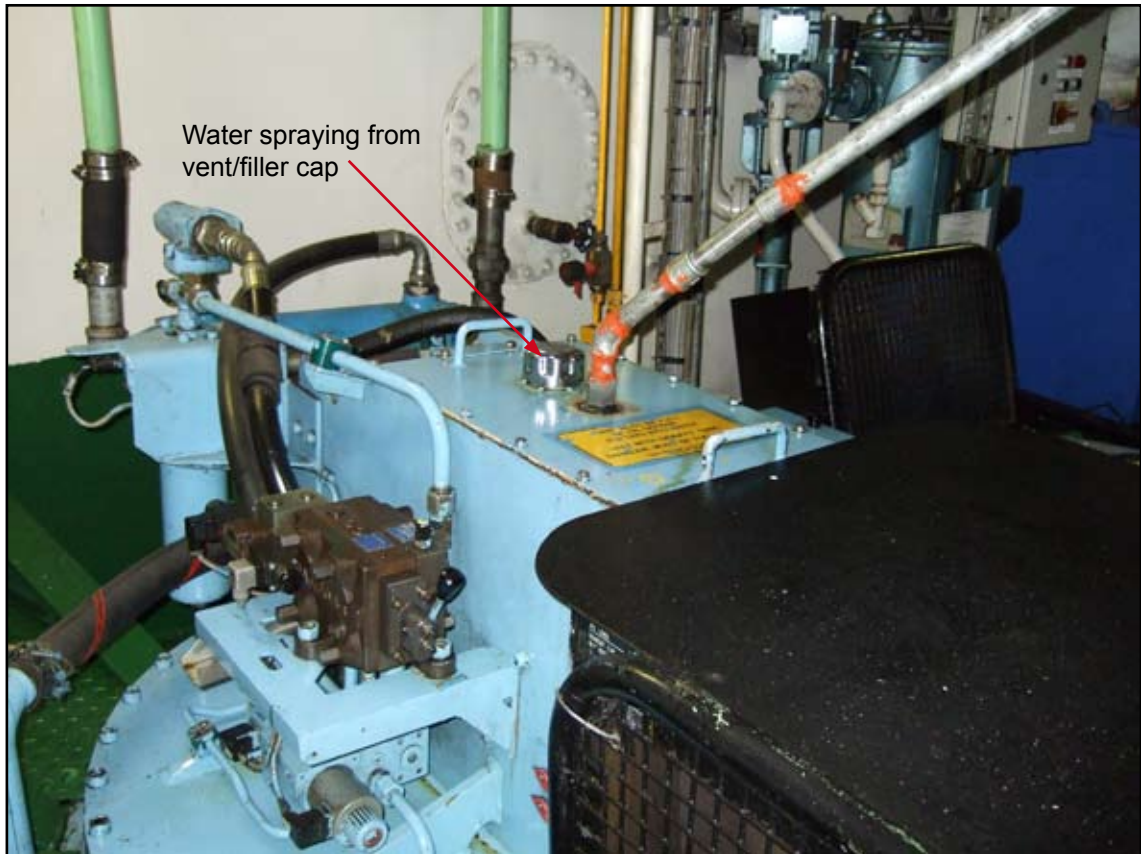
Photograph showing position of water ingress
