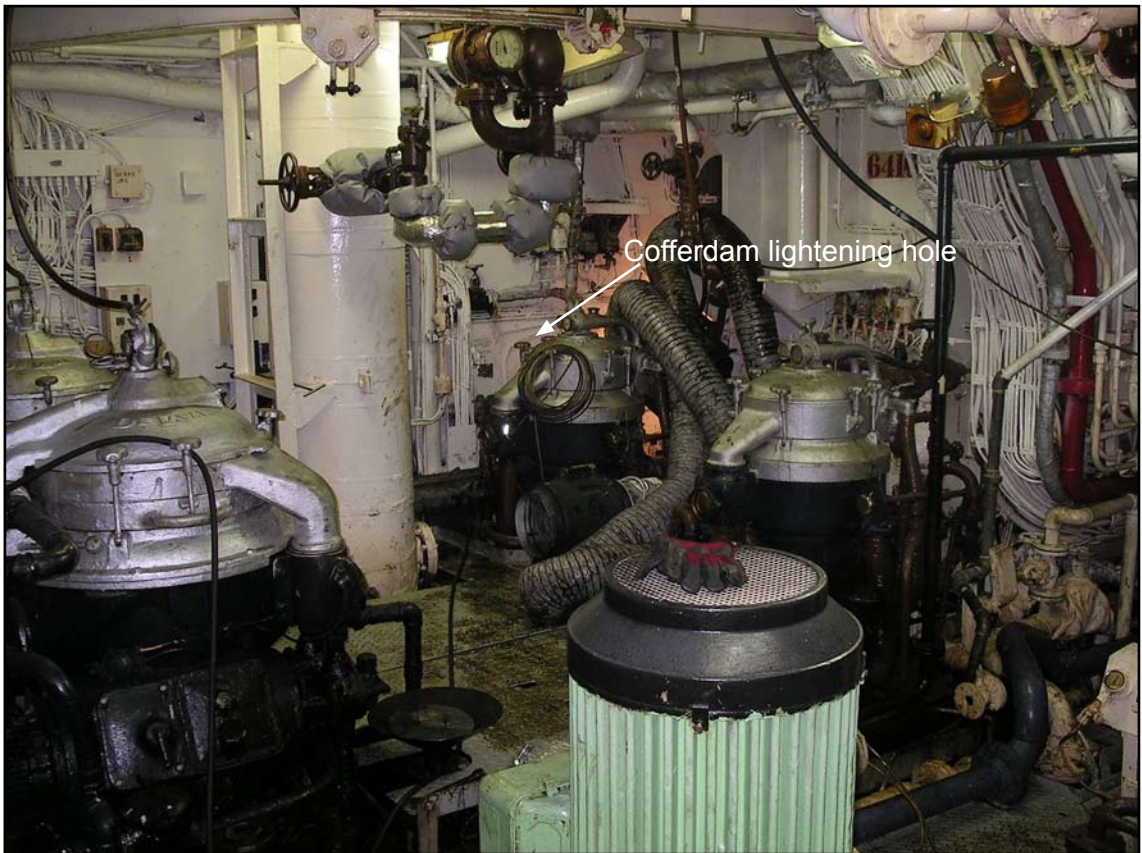
The purifier room
