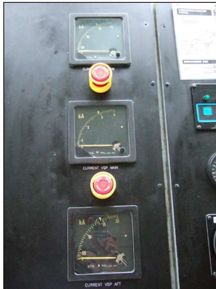
Ammeters on bridge control panel
