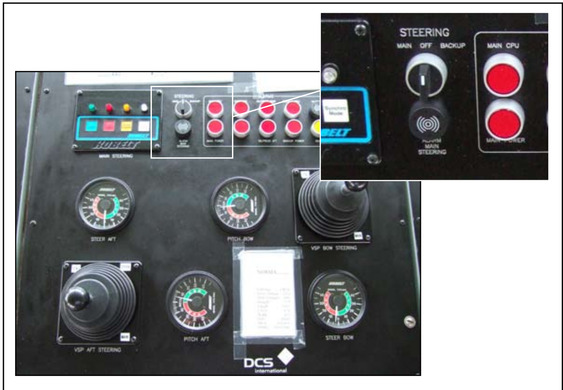
Propulsion and steering control panel
