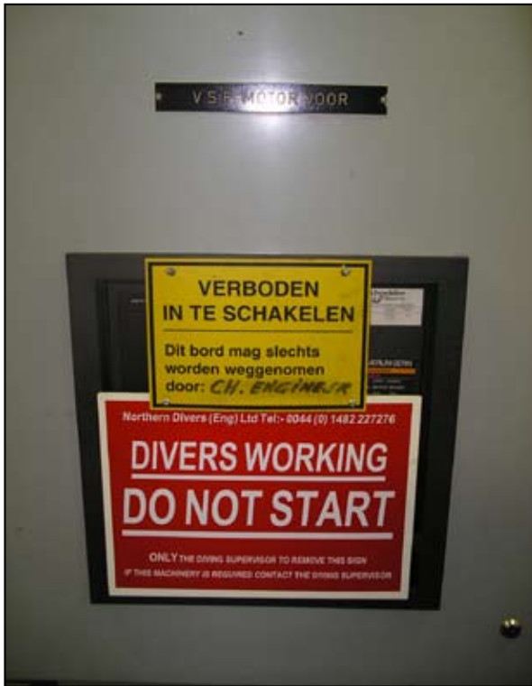
Warning sign on VSP switchboard
