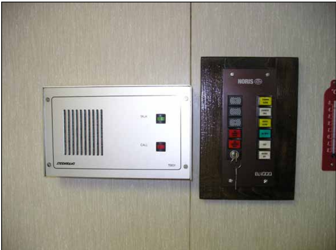
Watch alarm repeater in master's cabin
