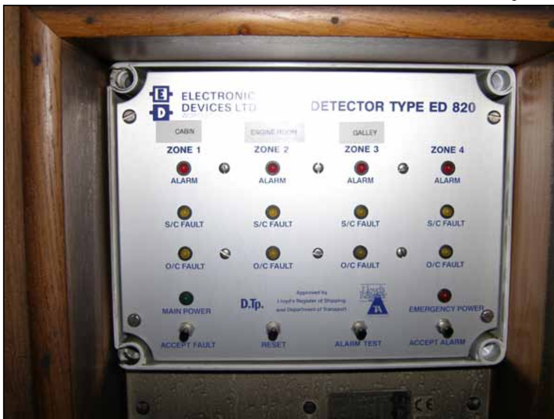
Fire detection panel
