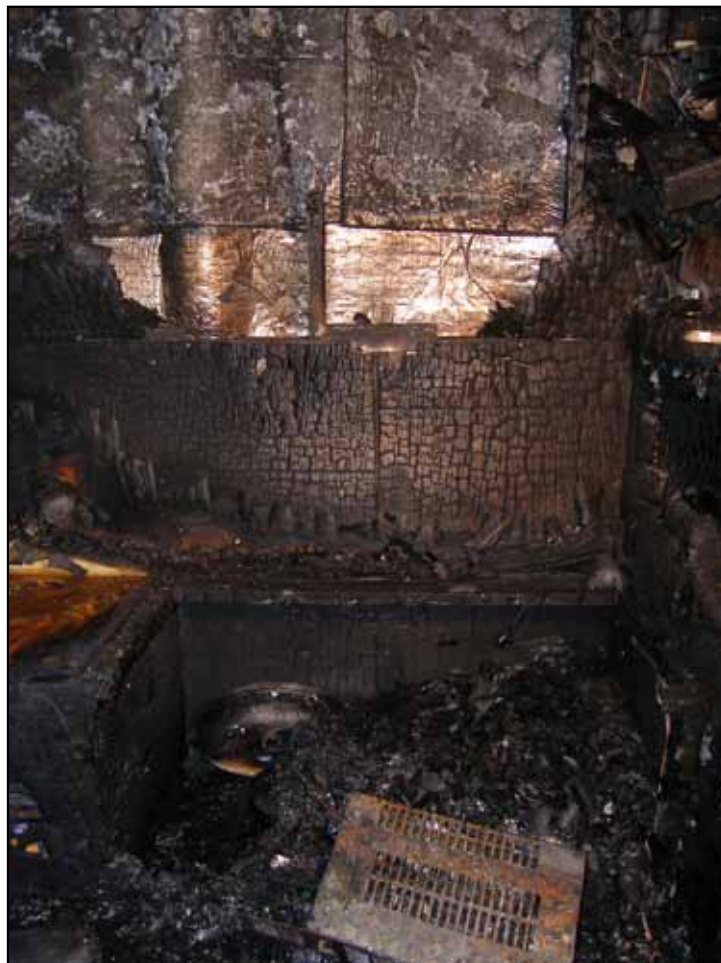
Seat of the fire in the vicinity of the electric heater
