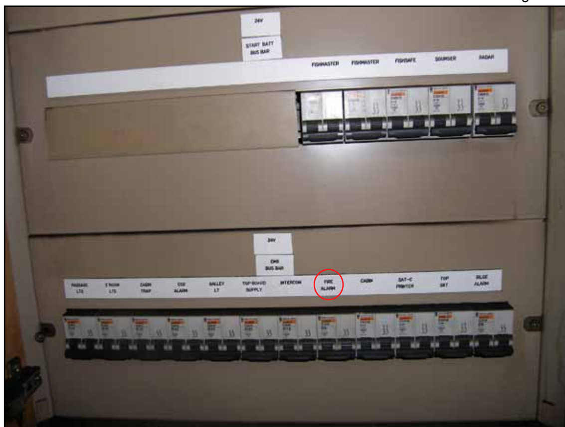
All equipment on the emergency bus bar turned off
