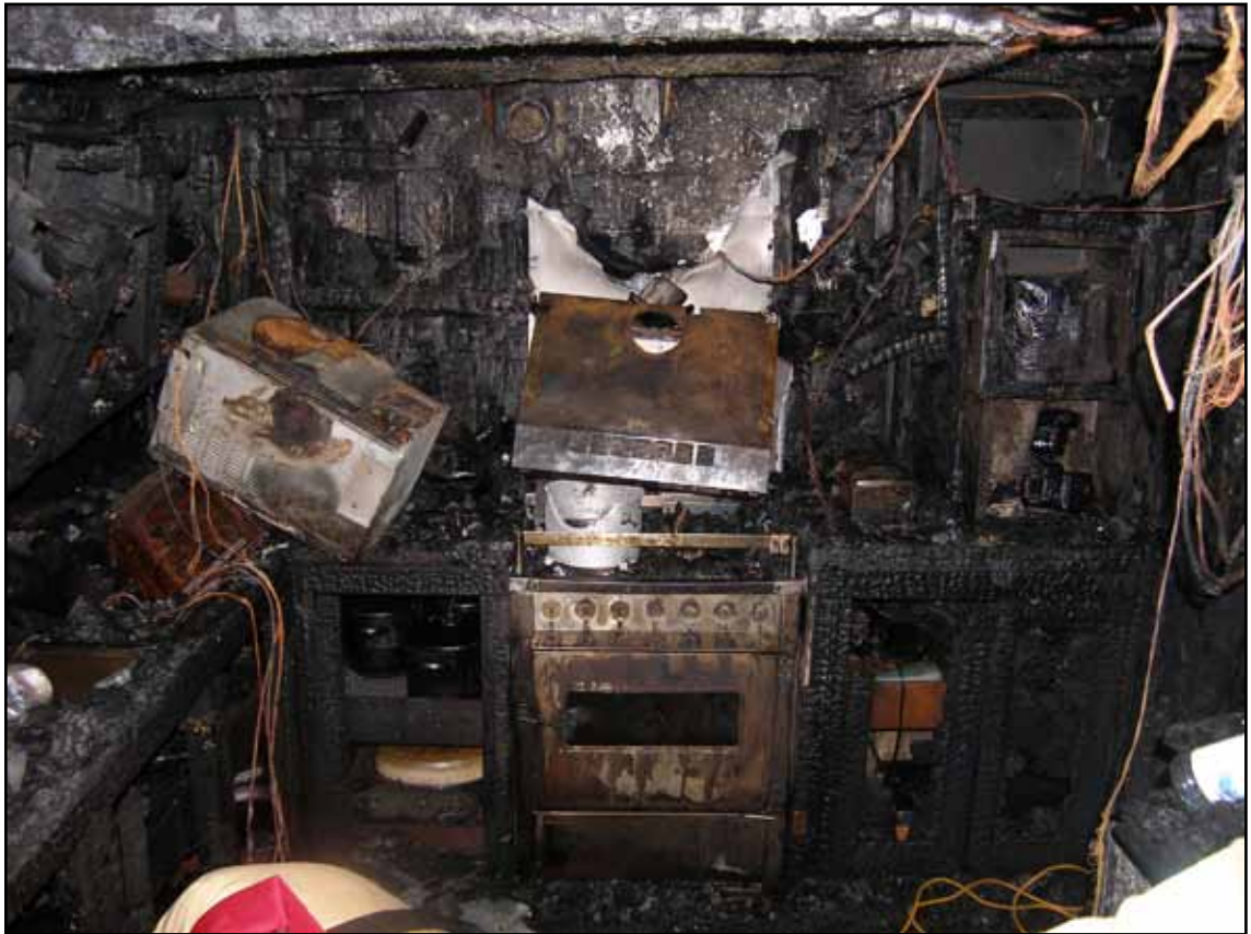
Galley range showing partially melted pan
