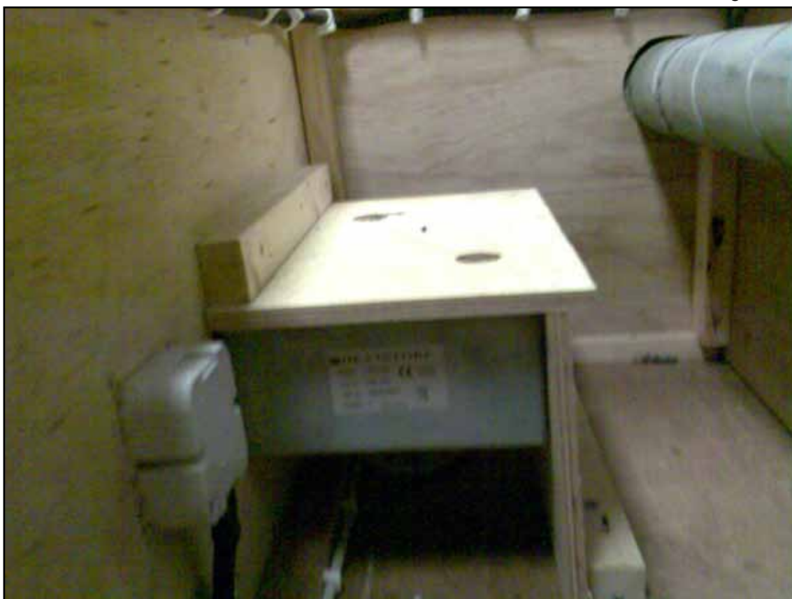
Partial 'boxing in' of heater on new vessel subsequent to this accident
