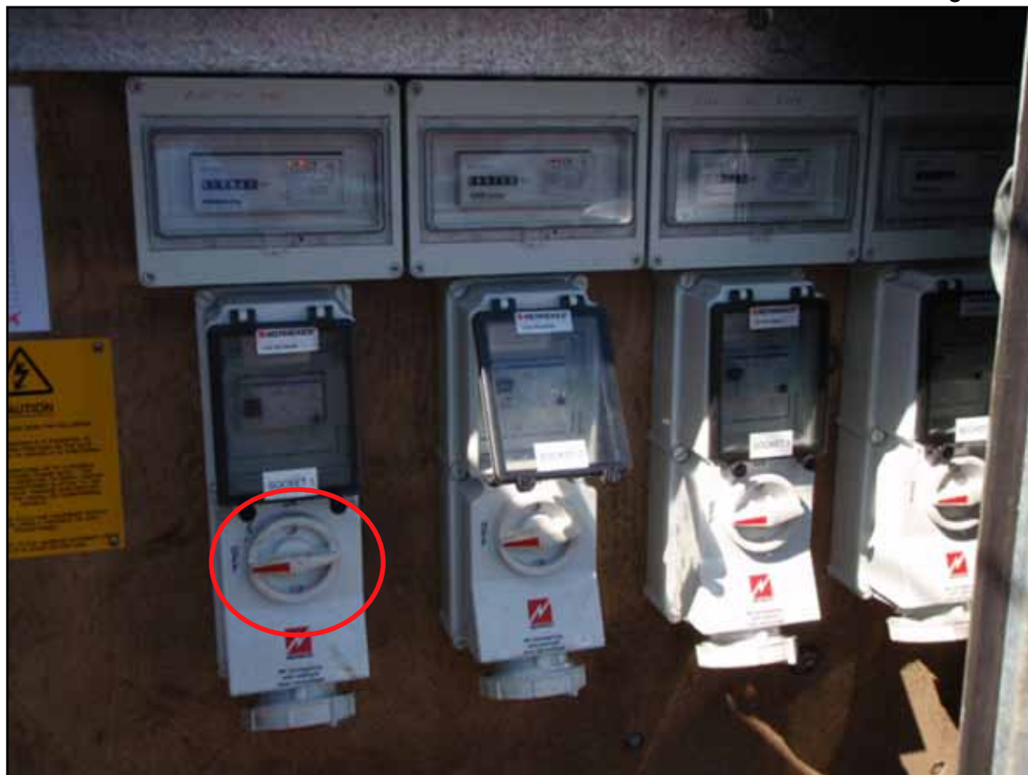
Shore power supply - Provost Park Jetty
