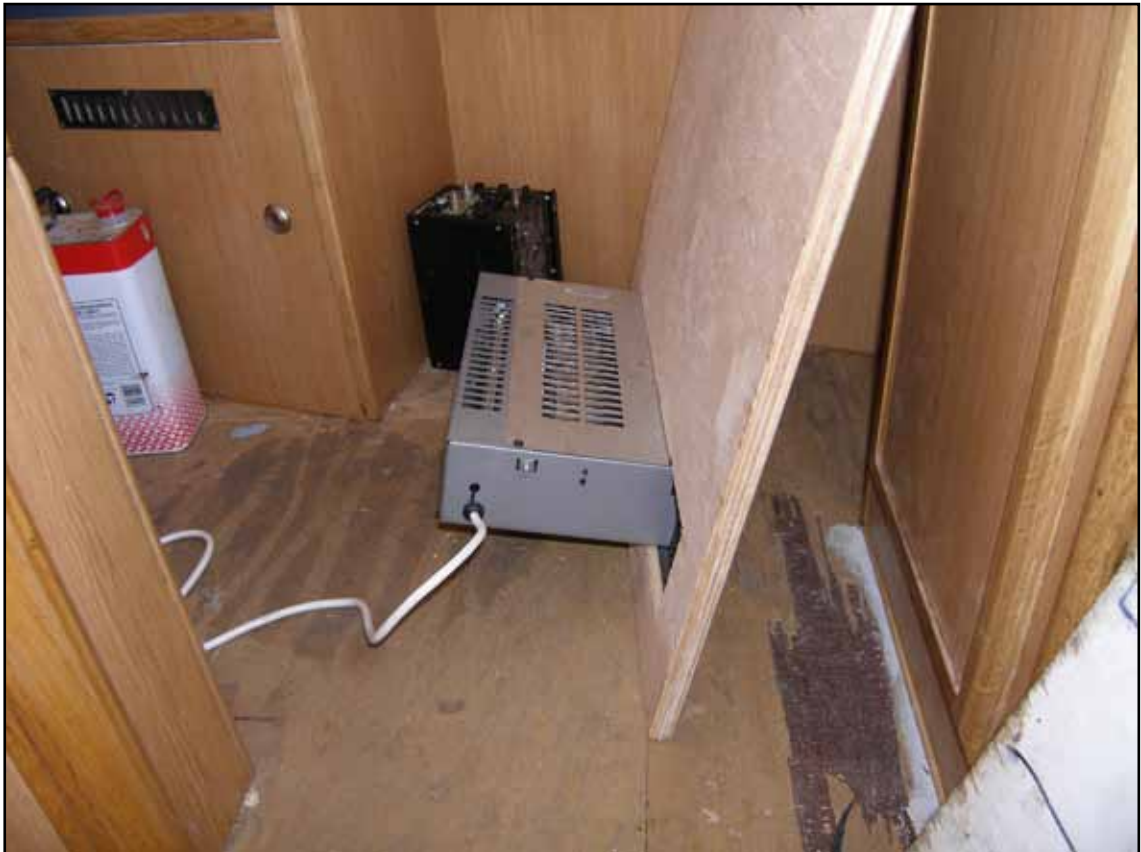
Heater positioned through the aperture
