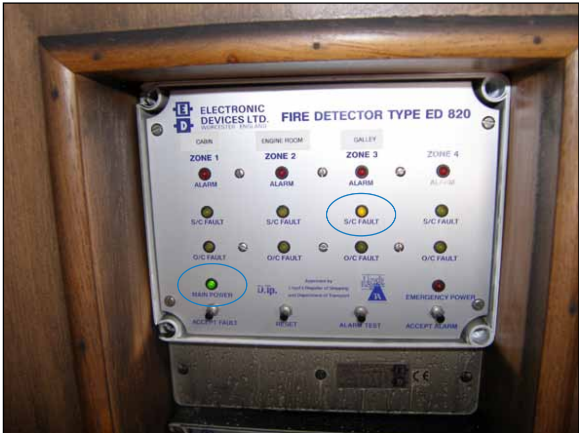
Fire detection panel activated by switching on fire alarm breaker
