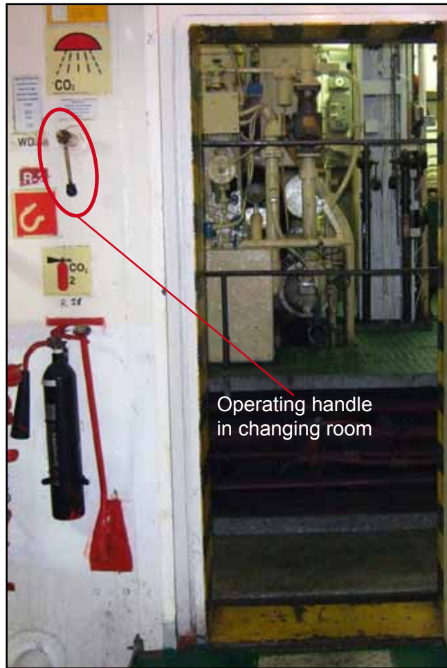
Photograph showing door operating handle
