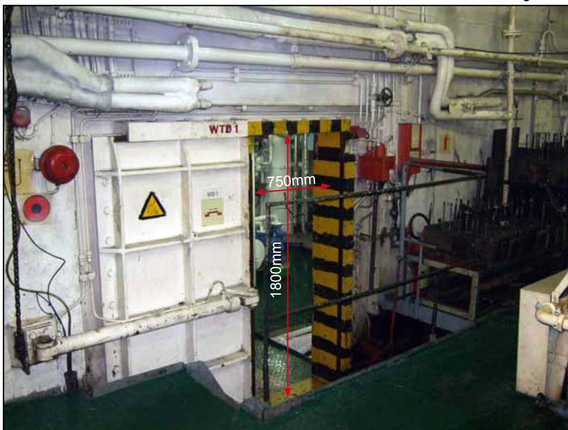
Photograph of watertight door No.1 (open) - view from auxiliary engine room
