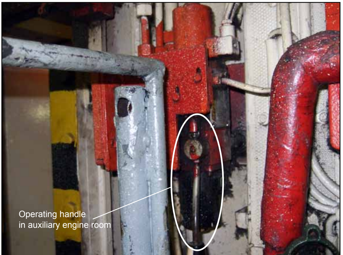
Photograph showing door operating handle
