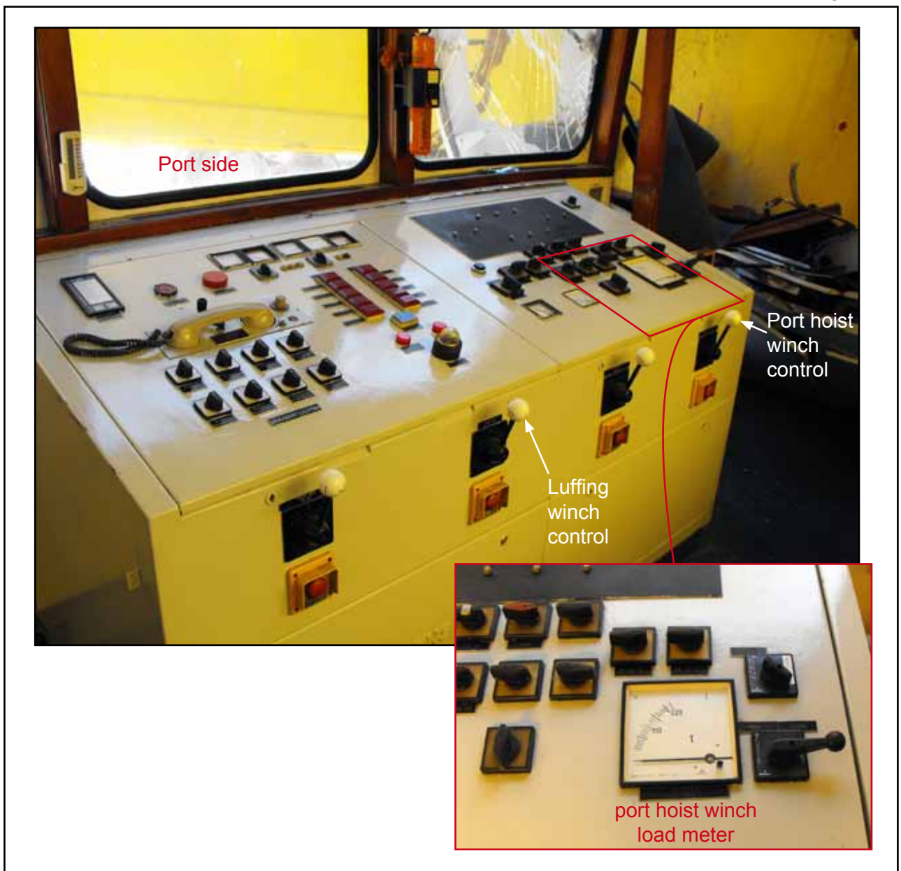
Control for port hoist winch and luffing winch control
