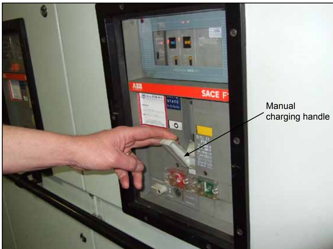
Main circuit breaker
