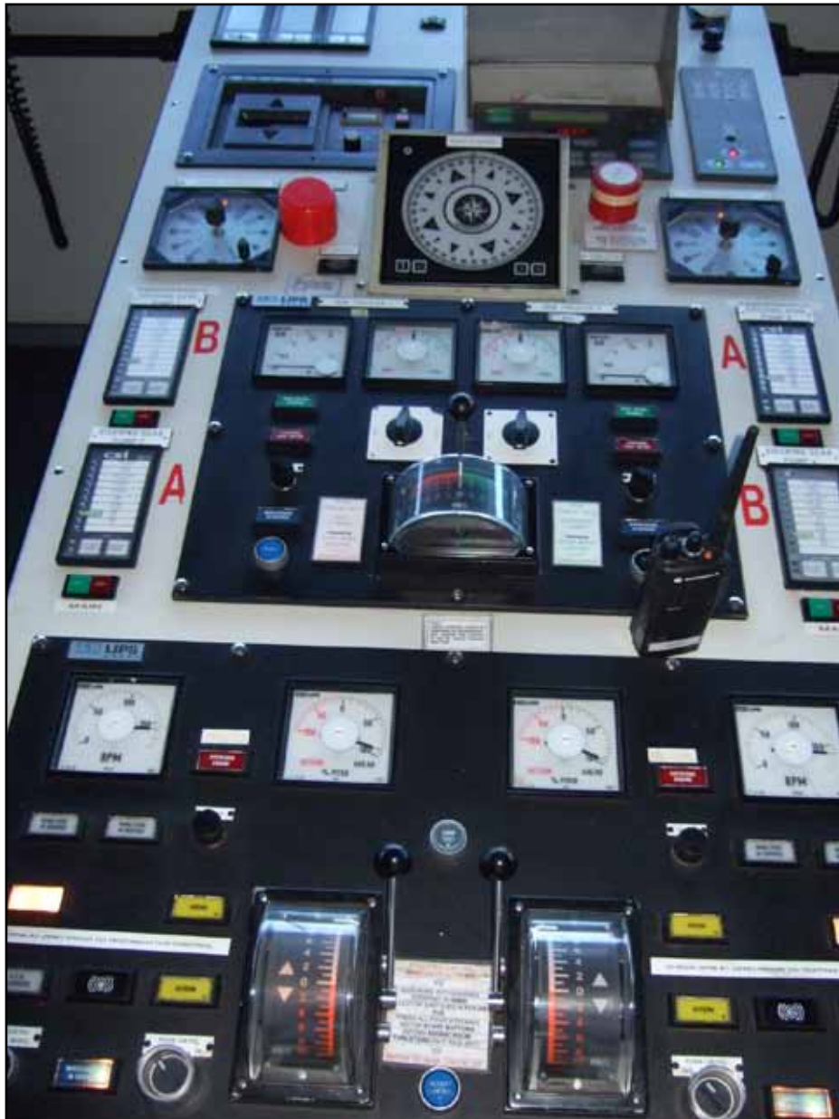
Centre control panel (bridge), looking down
