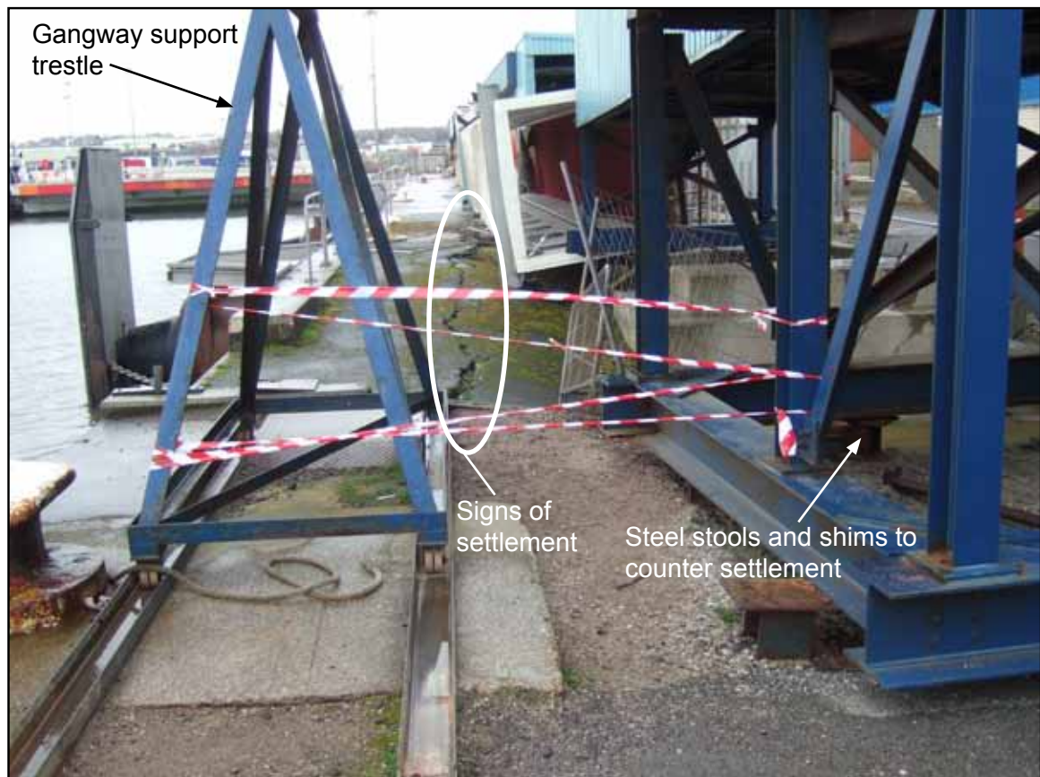
Gangway compartment support and settlement
