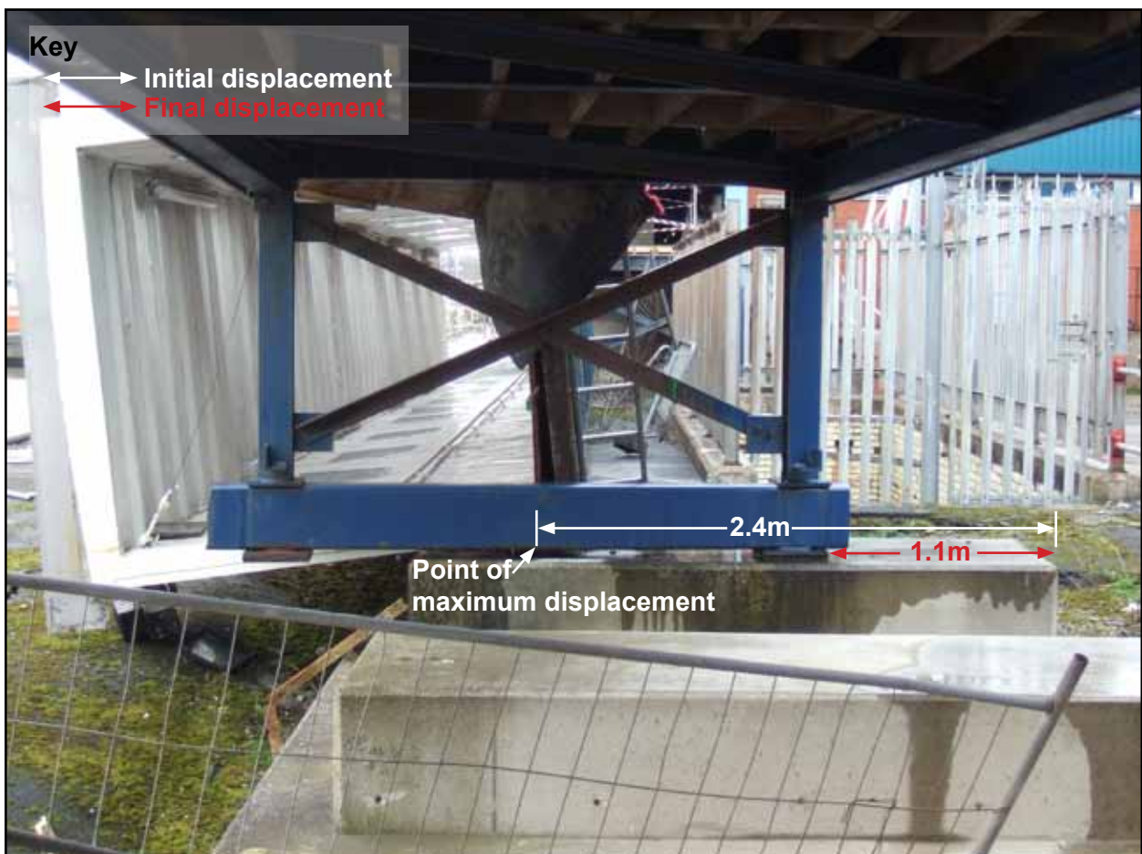
Movement of gangway compartment showing support frame in its final position after the accident
