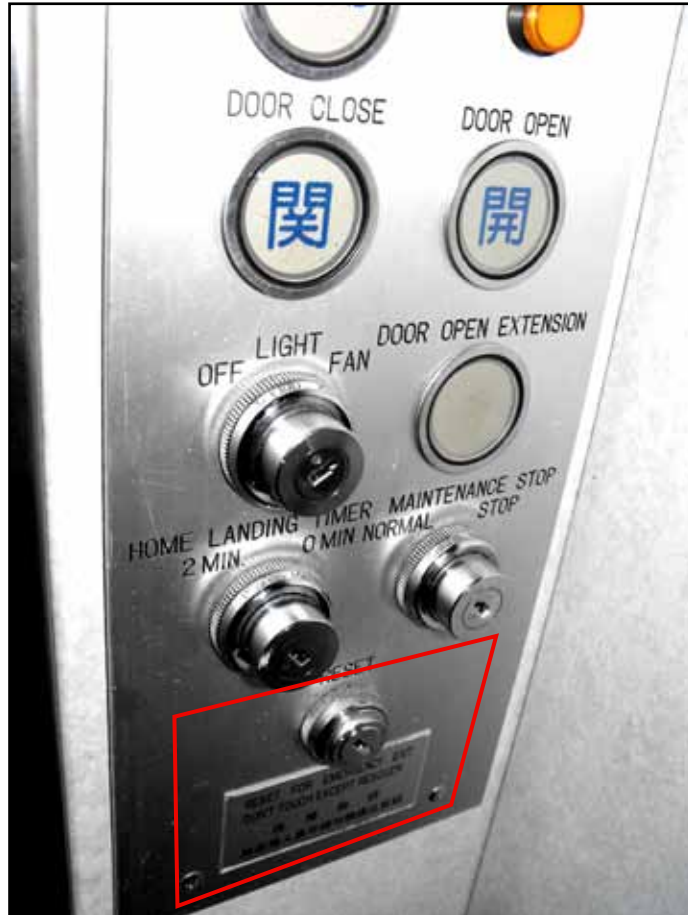
Lift reset switch - located in lift car
