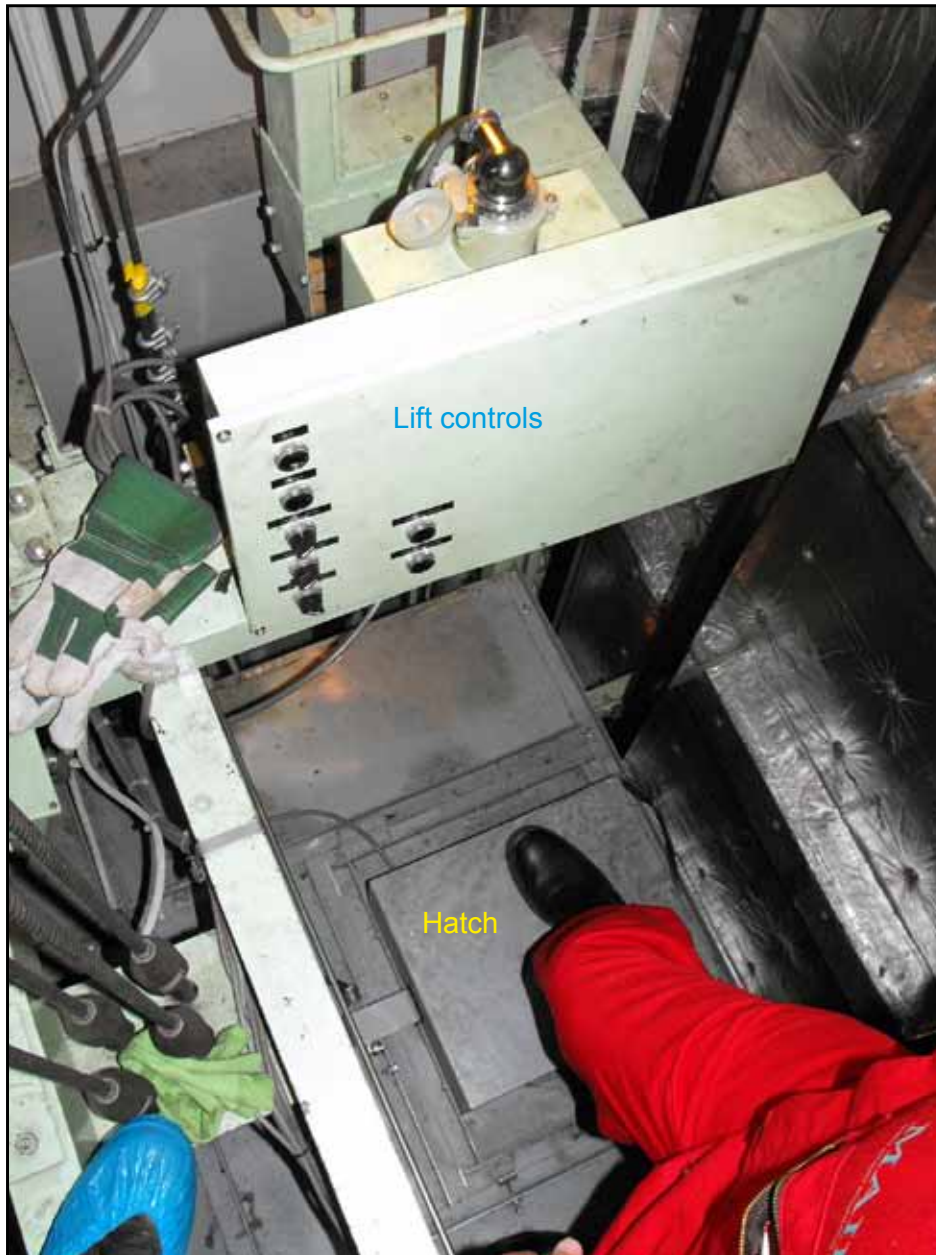
Lift car emergency escape hatch and local control switches
