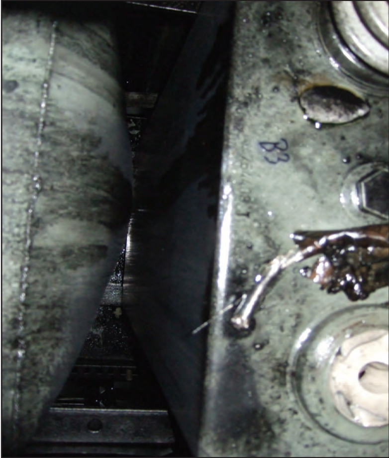
Top view of bulged capacitor
