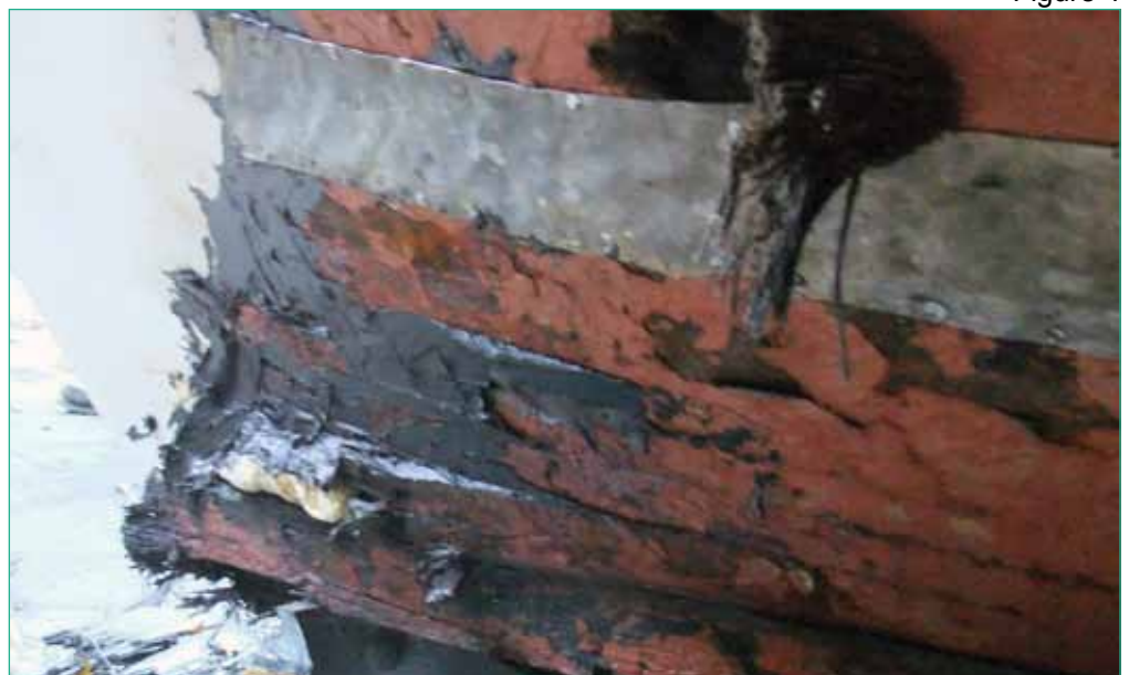
Stem post damage
