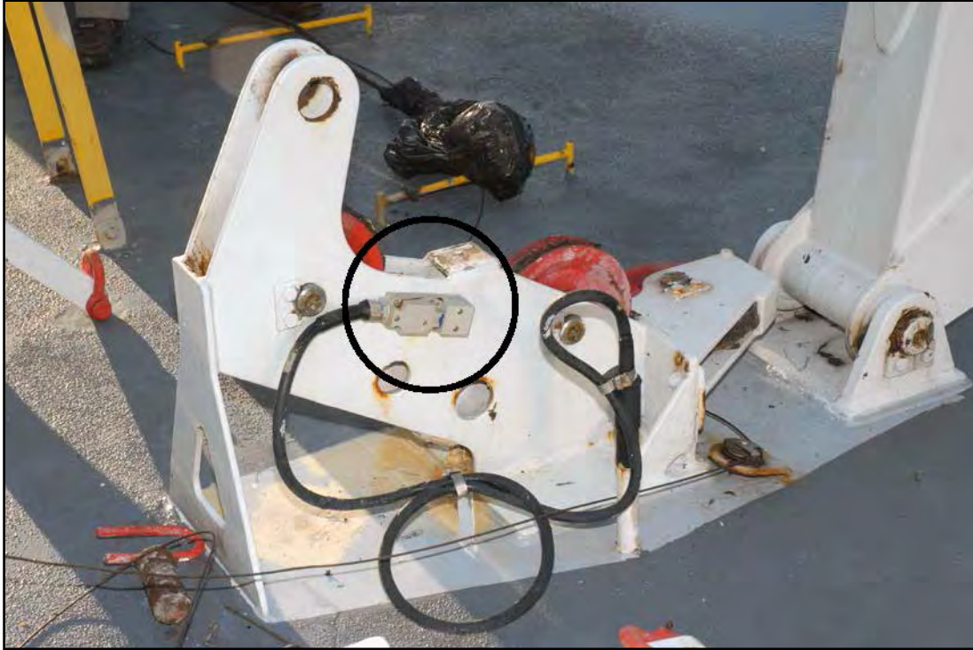
Figure 2: Proximity switch on davit (circled)
