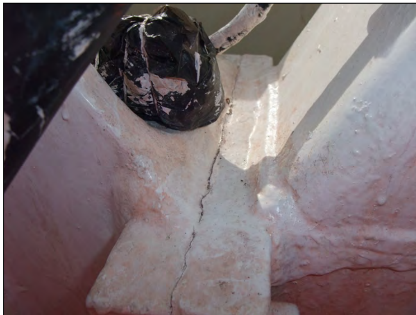
Figure 14: Cracked paint indicating movement between wheel unit and crane ( Blue Carmel )
