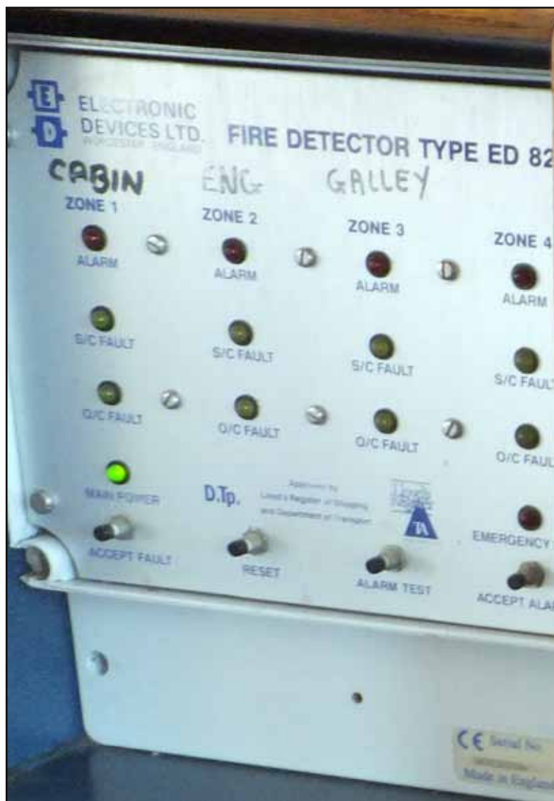
Figure 6: Fire detection system control panel ( Ocean Challenge )
