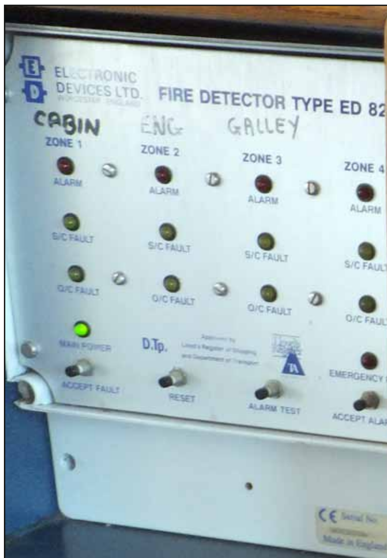
Figure 6: Fire detection system control panel ( Ocean Challenge )
