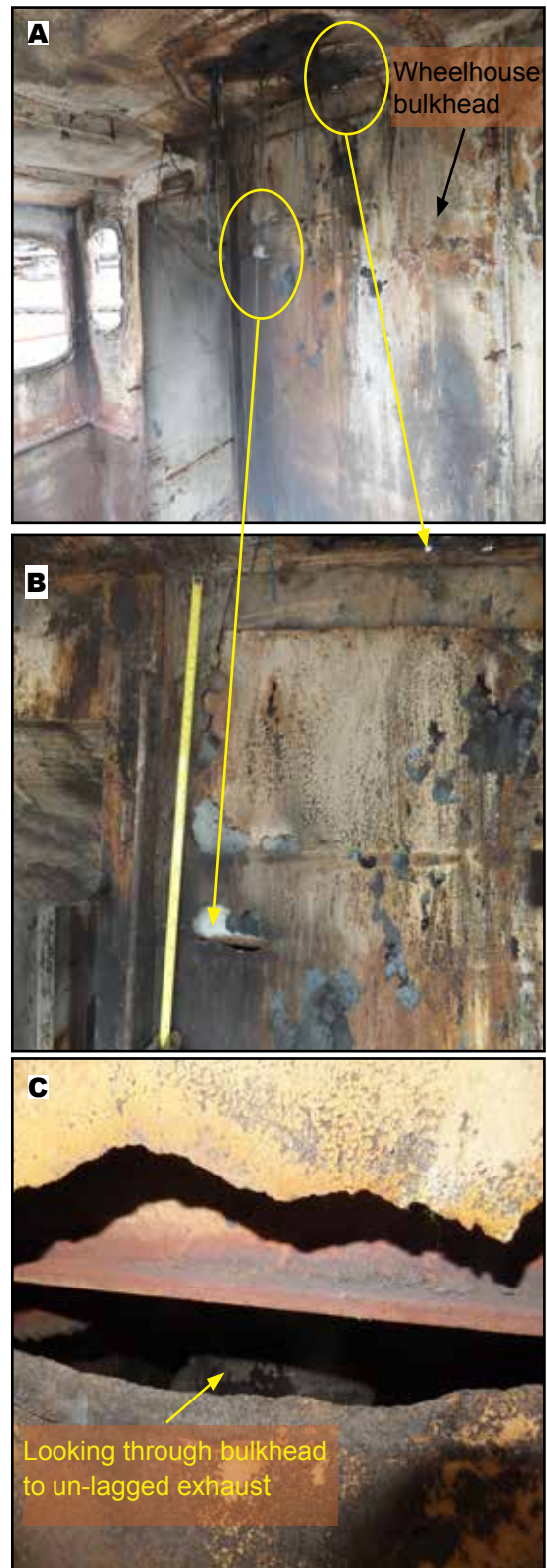
Figures 4a, 4b and 4c: Showing corroded bulkhead damage
