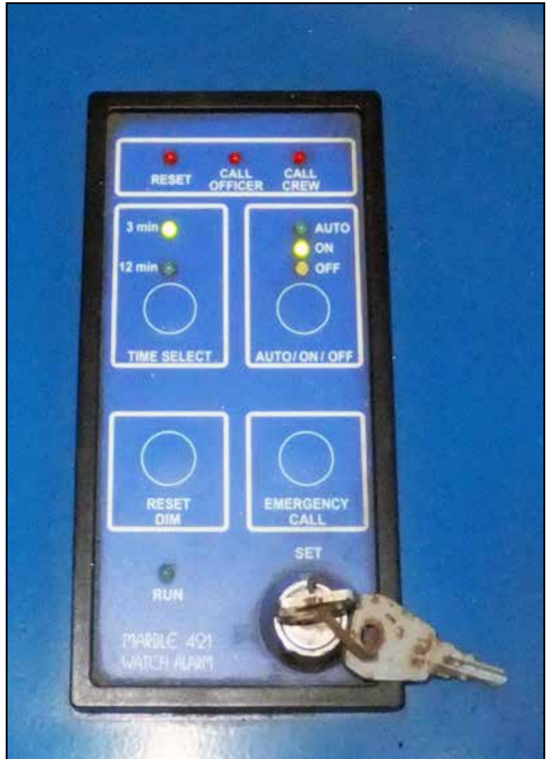
Figure 2: Bridge navigation watch alarm system's control
