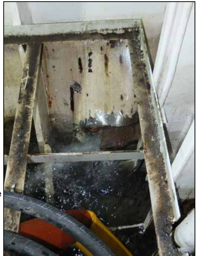
Figure 4: Hull shell penetration in pump room
