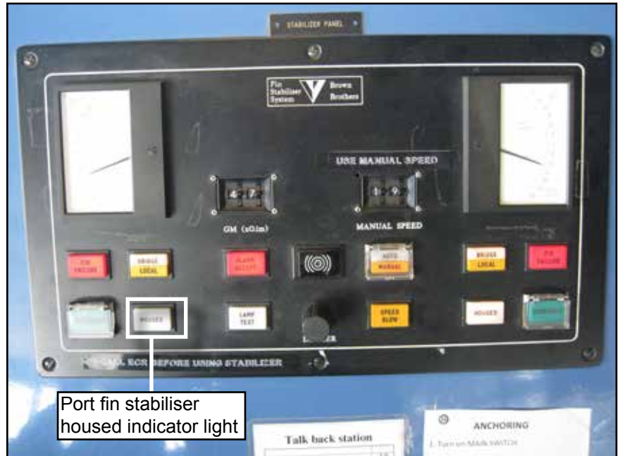
Figure 7: Fin stabiliser panel on the bridge centre console
