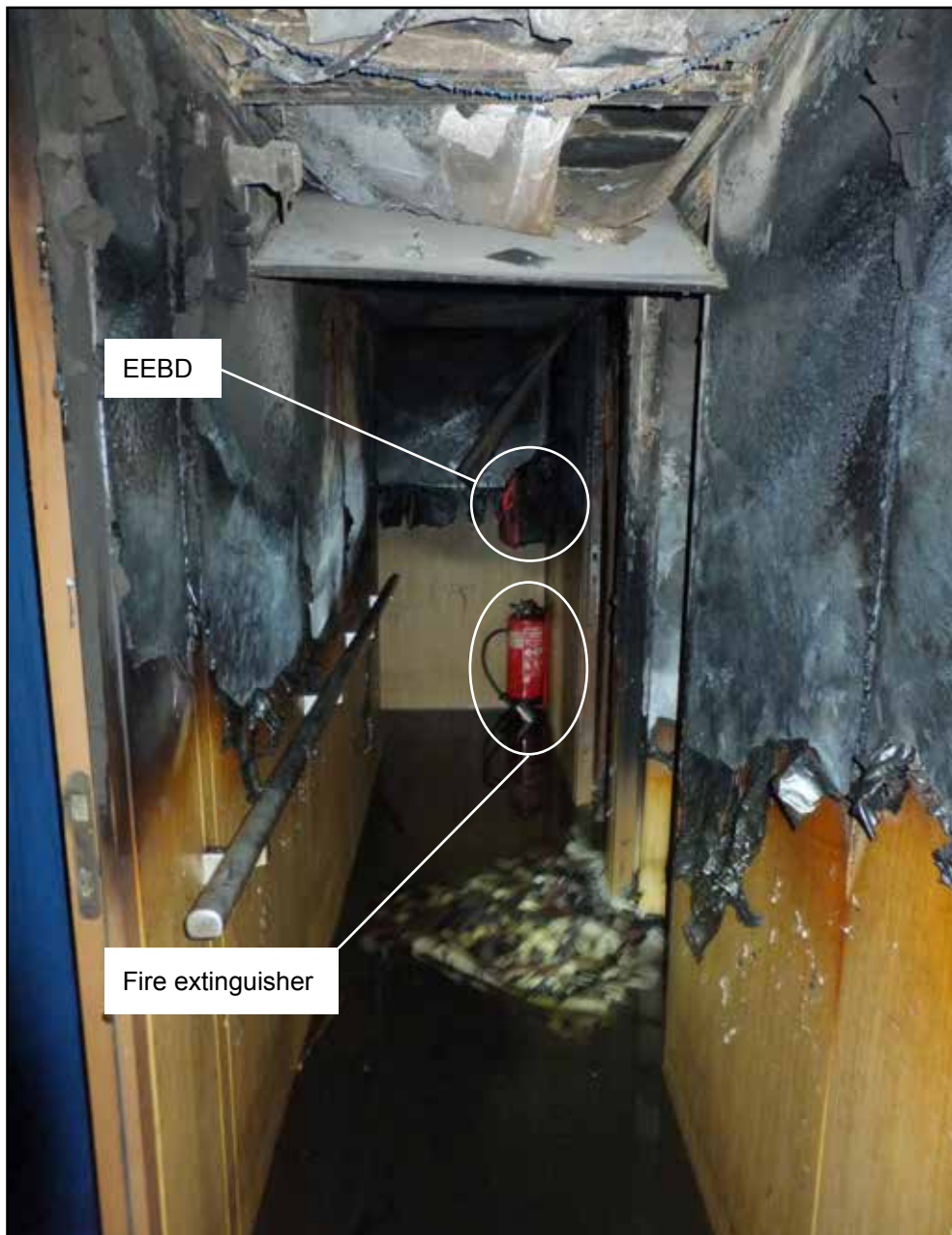
Figure 16: Deck 2 starboard alleyway - post fire showing fire extinguisher and EEBD
