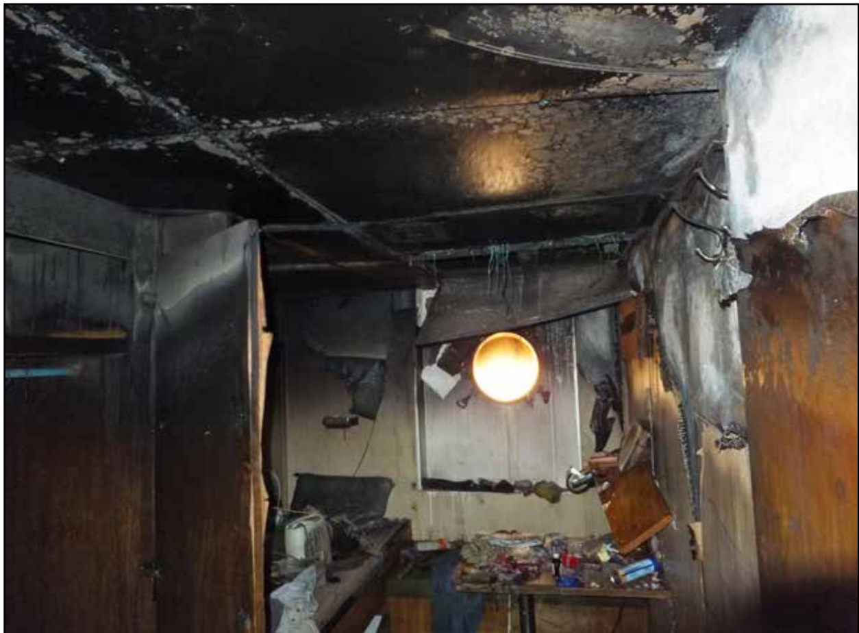
Figure 10: AB1's cabin - post fire
