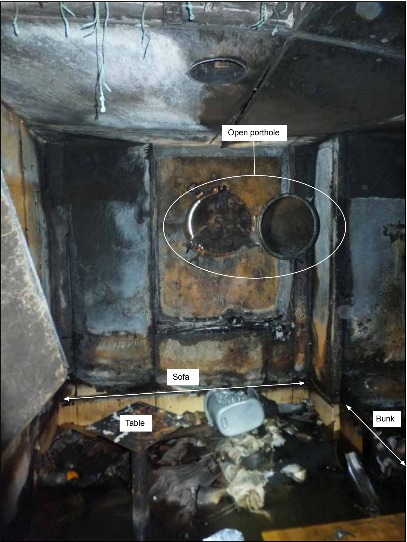
Figure 8: AB2's fire-damaged cabin
