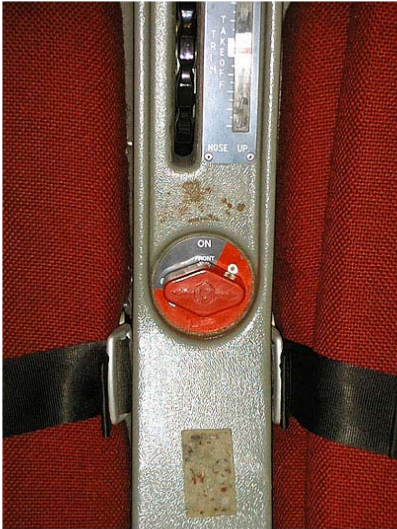
Figure 2 - Fuel ON/OFF cock in G-RAFA (Note position relative to elevator trim wheel)
