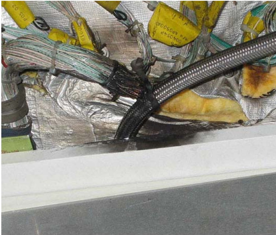
Figure 1 Damaged loom and hose, G-DOCH
