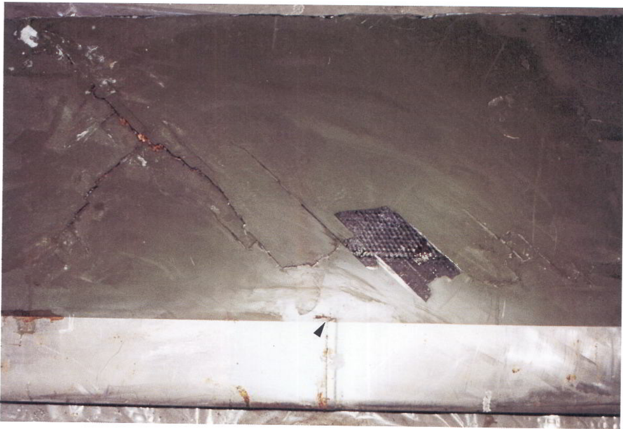
Figure 9A: Showing localised blade skin damage at overlap of leading edge anti-erosion shield sections due to related arcing on 'Black' MRB.
