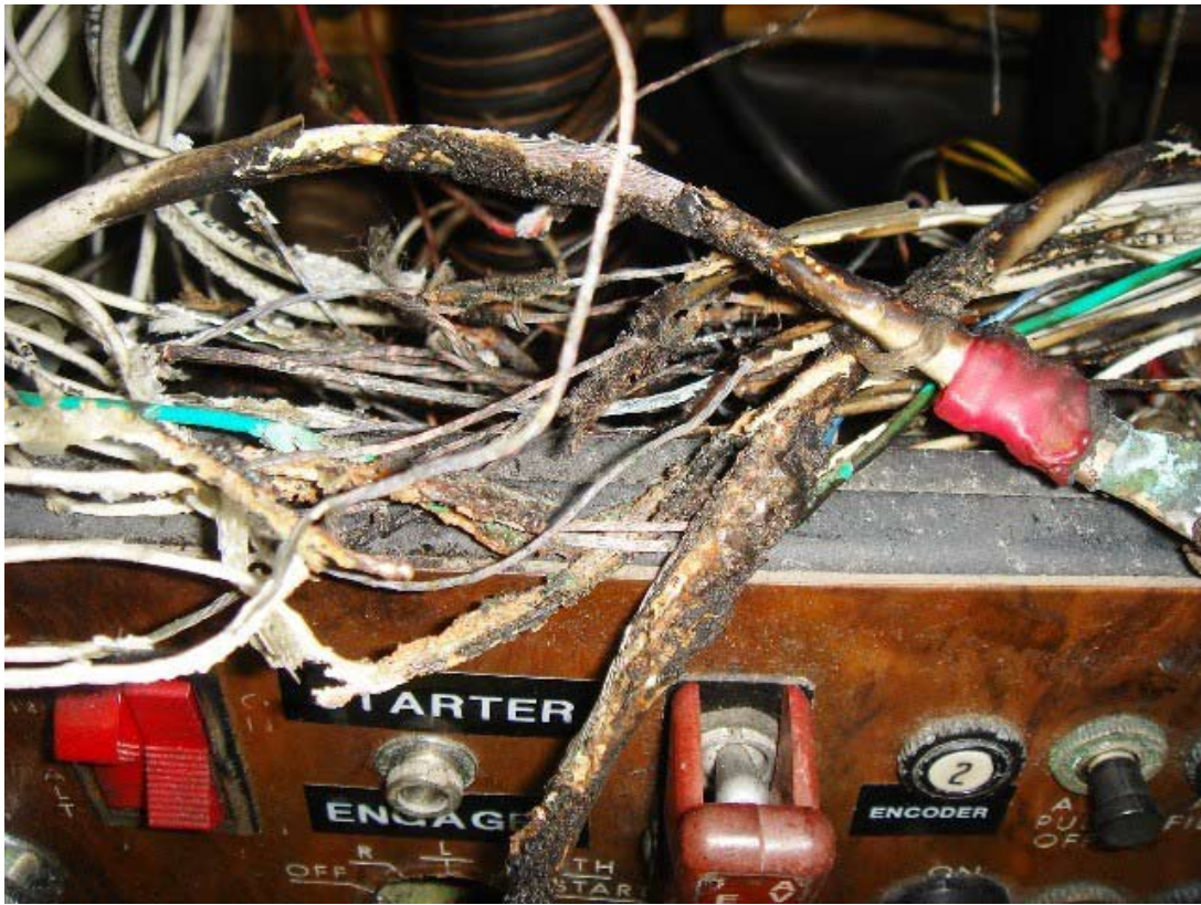
View of wiring damage
