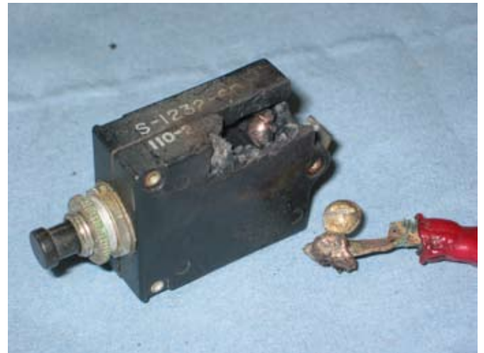
Alternator circuit breaker and feed wire
