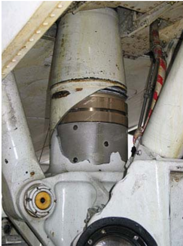
Nose landing gear outer cylinder showing the area from which the ejected section of cylinder material originated
