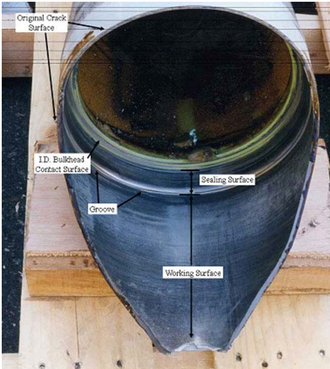
Nose landing gear outer cylinder that was involved in the 1998 incident showing the area of failure (Photograph courtesy of Boeing Materials Technology)
