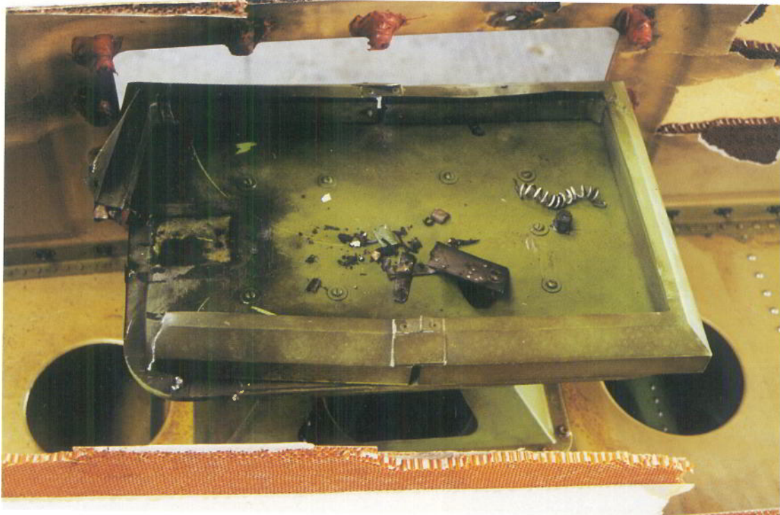
Photo 3 Damage to antenna assembly. (Small debris retrieved from inside fin top structure)
