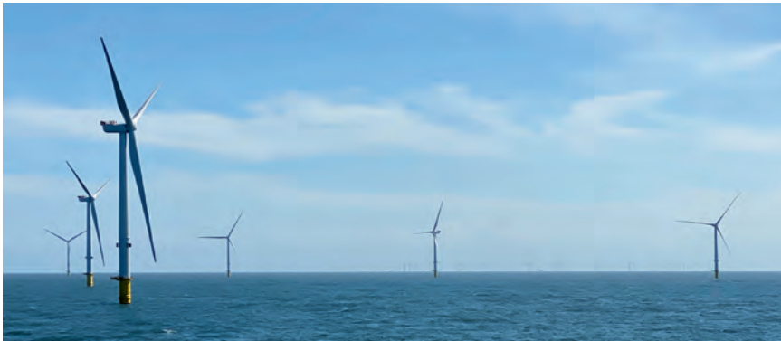
Above: Triton Knoll wind farm began turbine installation and achieved first generation in 2021.
