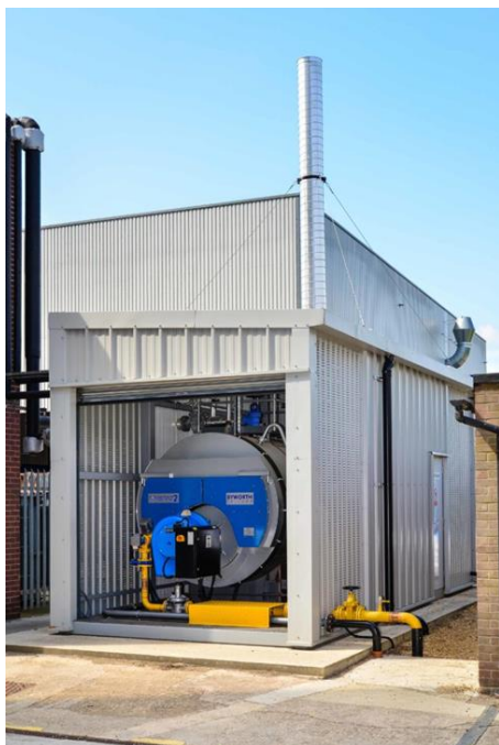
Figure 4. Limpsfield co-firing burner unit (Image from (Limpsfield, 2020)).
