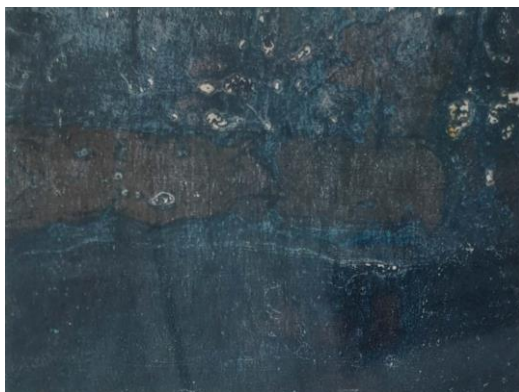
Figure 1-2 Rust Grade A
