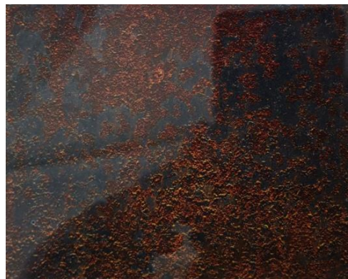
Figure 1-3 Rust Grade B
