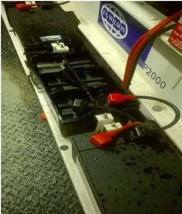
Photograph – 01: A3 Generator Plantroom (Battery No 2). Point of Explosion.
