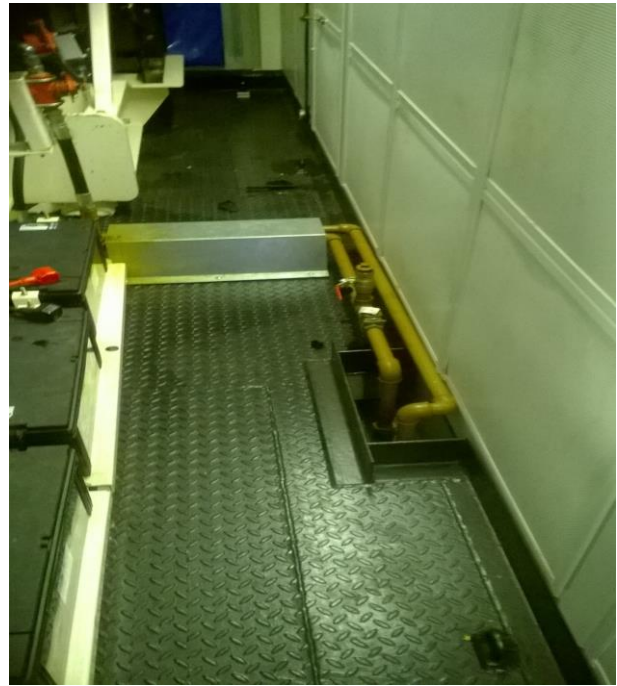
Photograph – 02 : Photograph shows extent debris was deposited within the generator room. Note: Plastic battery casing at front of generator opposite side approximately 4 Metres from discharge point.
