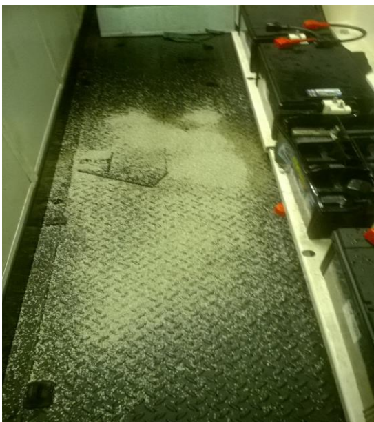
Photograph – 03 : Photograph shows extent debris was deposited within the generator room. Note: Plastic battery casing to side of generator adjacent to discharge point.
