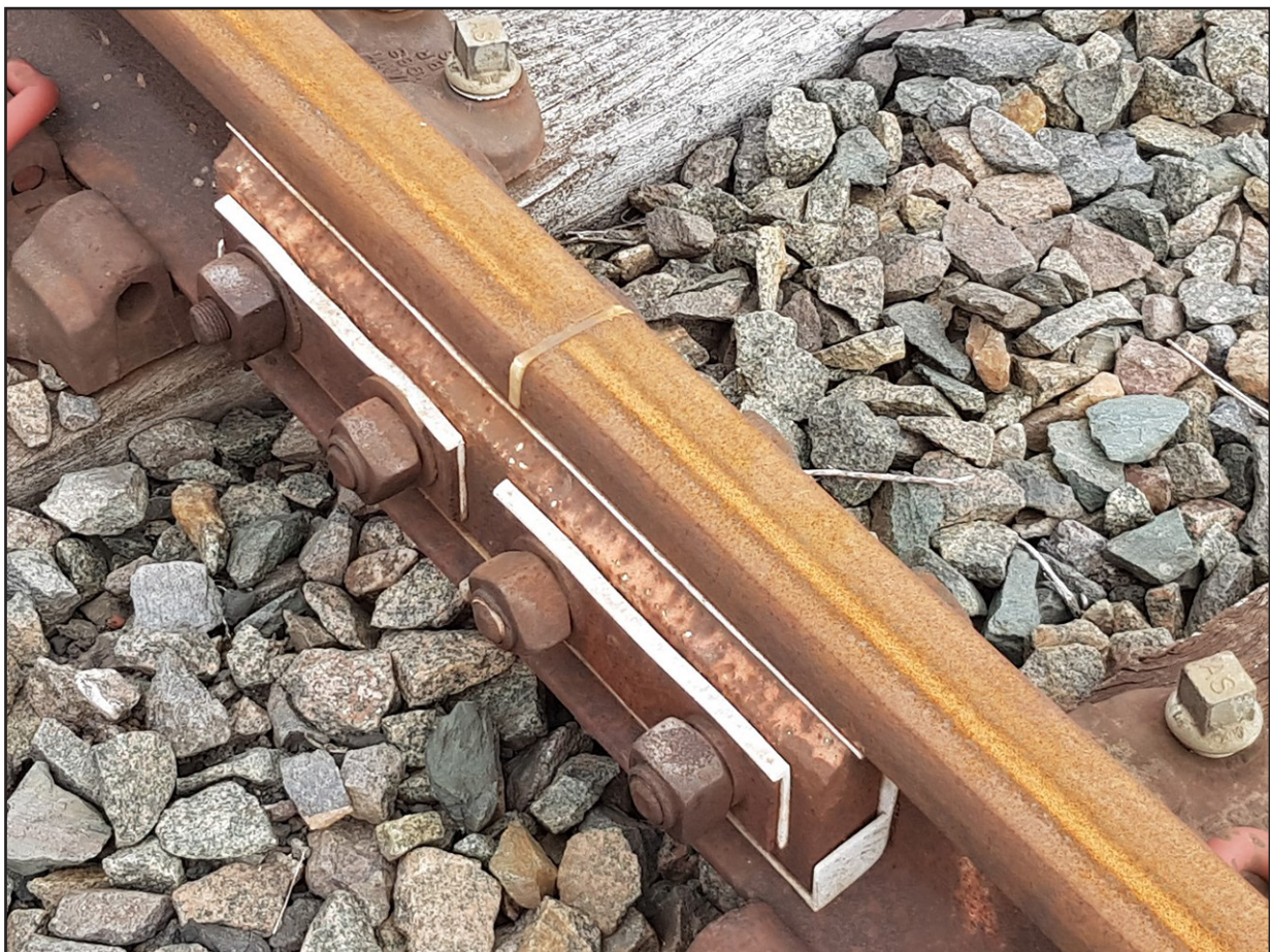
Figure 6: Insulated rail joint
