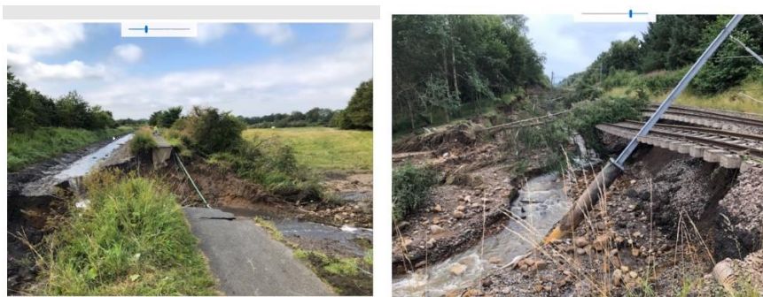
Figure 6: Interdependencies: The Union canal embankment collapse washed away the railway between Edinburgh and Glasgow (12 August 2020)
