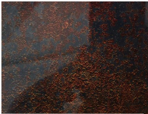
Figure 1.3 Rust Grade A
