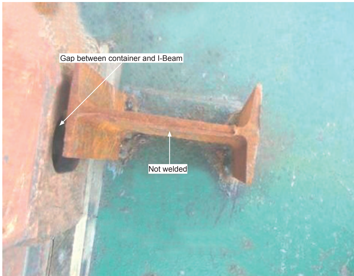
Figure 1: Poor quality welding
