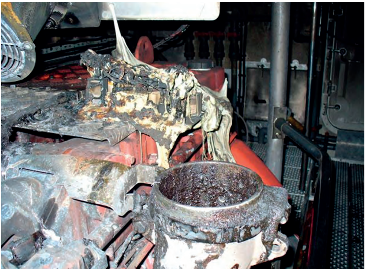
Figure 4: Damage to plastic fitting
