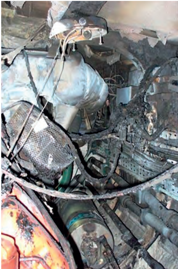
Figure 3: Electrical cable damage
