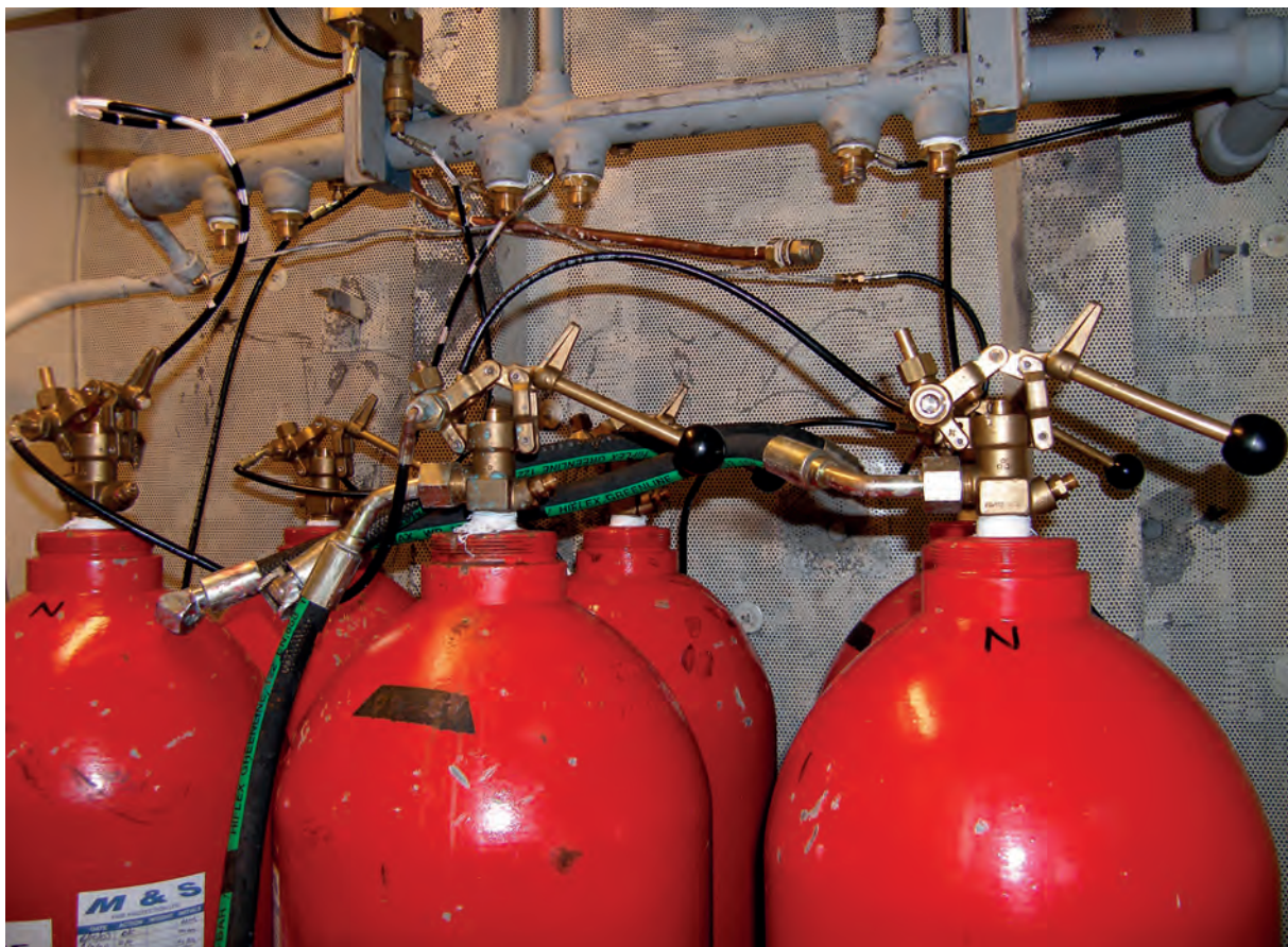
Figure 2: The disconnected hoses
